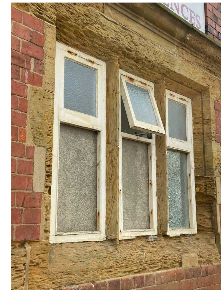
Example of Window and Stone Surround Condition
