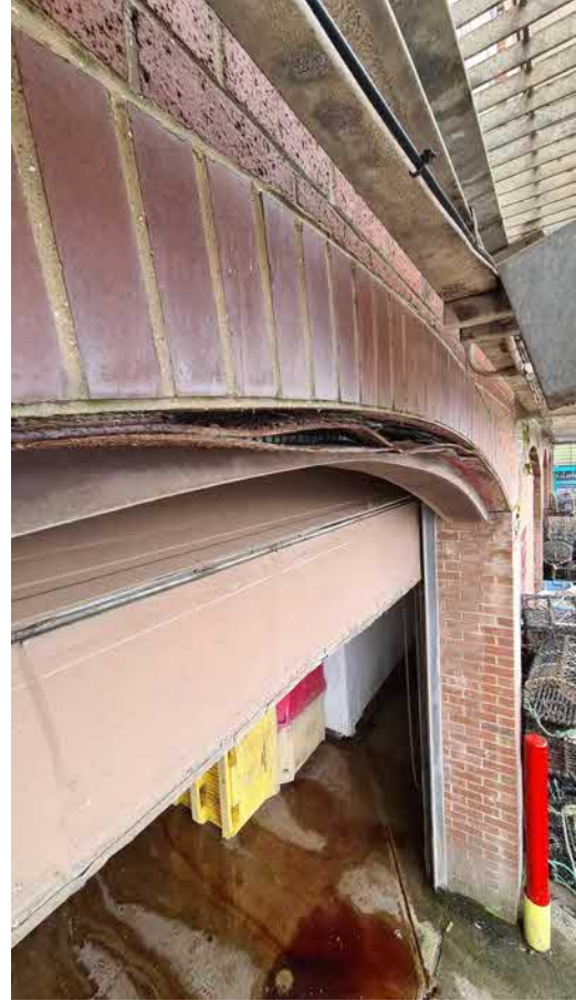
Figure Steel Lintel distortion & flashing separation
