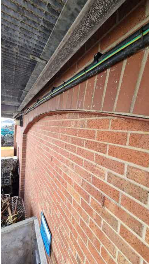
Figure Steel Lintel distortion
