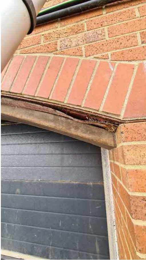
Figure Steel Lintel distortion & flashing separation
