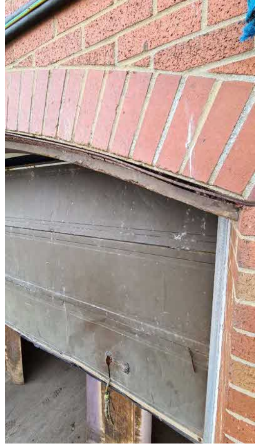
Figure Steel Lintel distortion
