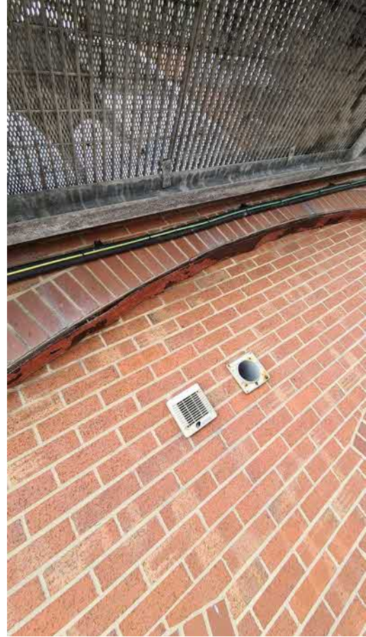
Figure Steel Lintel distortion
