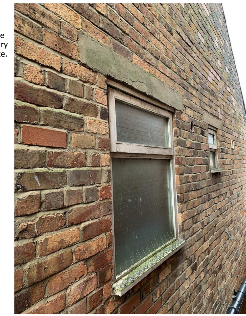
Windows and Lintels to be replaced to SE Elevation
