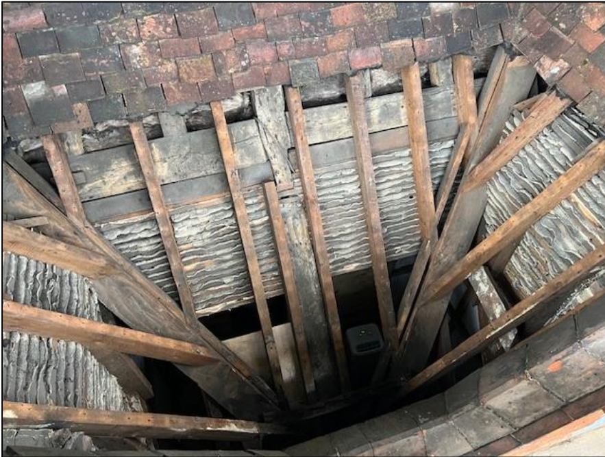
Figure 5 – Image showing the area of roof in need of repair ©National Trust.
