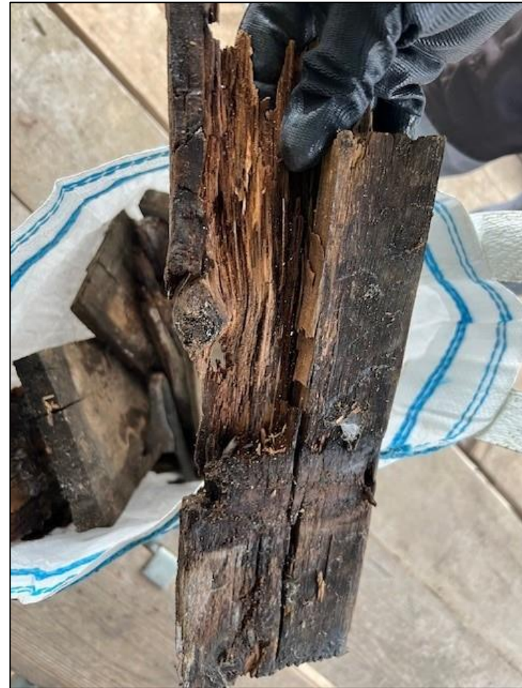
Figure 4 – Image showing a section of decayed timber from the roof ©National Trust.
