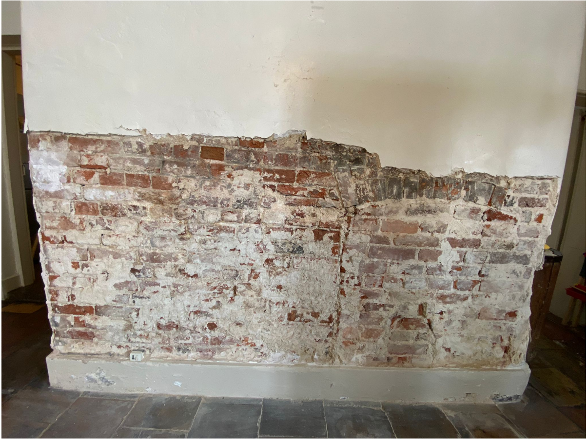
Image 1: Showing findings of investigation following removal of lime plaster, with existing fireplace shown to the right-hand side of the chimney breast
