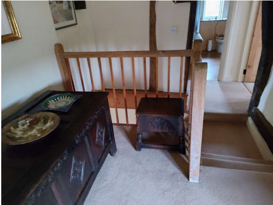
Figure 19; View of the first-floor landing showing the balustrade from the landing side.
