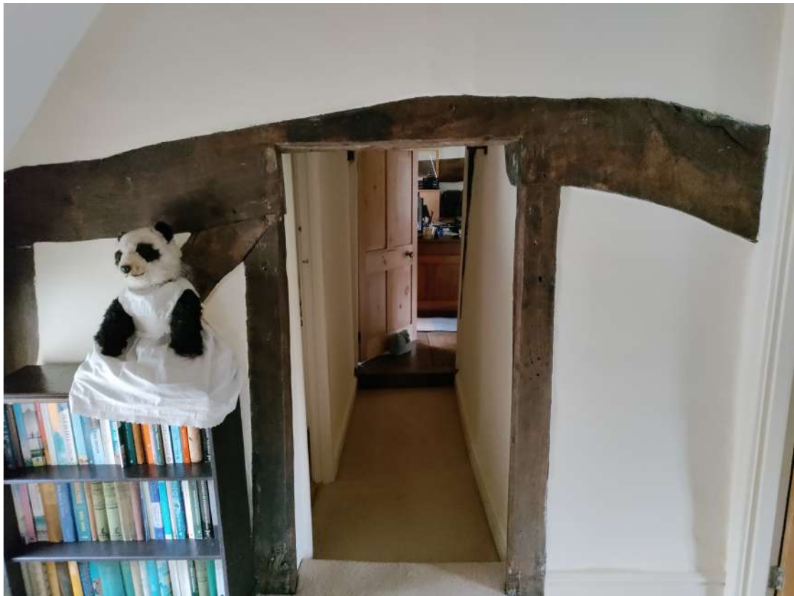
Figure 20; View of the tie beam leading through to the Easternmost bedroom, illustrating how low it is, even with the underside cut out.
