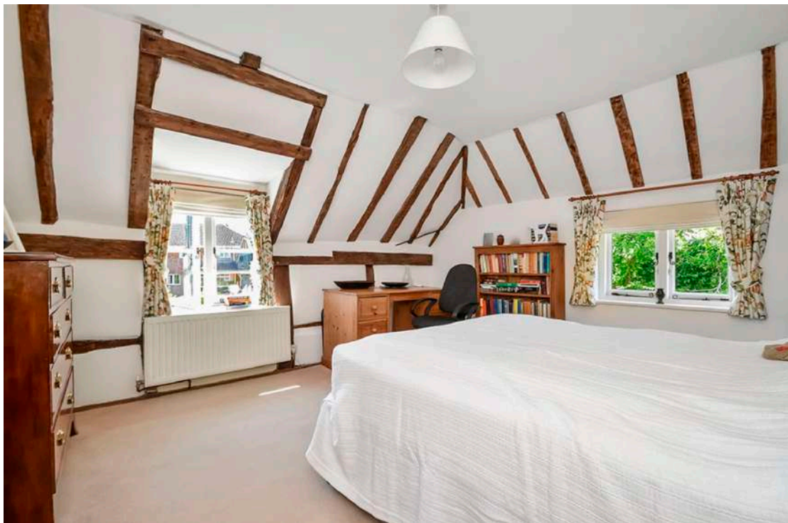
Figure 24; View of the South-Westernmost bedroom, within the C18 section of the farmhouse. Image by Knight Frank.
