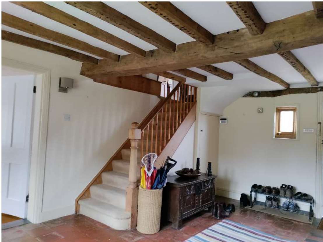
Figure 14; View of the existing staircase in the hall, showing the poor quality twentieth century softwood stair, newel post, and balustrade.
