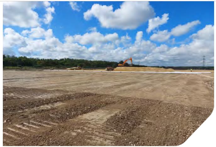
Photo 10: View of smooth rolled Zone 8 prior to CBR tests and piling mat extension
