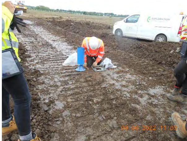
Figure 4. Scraped off area following compaction and sand replacement test being carried out.
