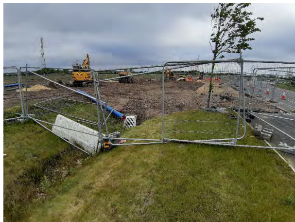
Figure 5. Inlet section between swale and transfer pipe adjacent to 278 works along International Drive.
