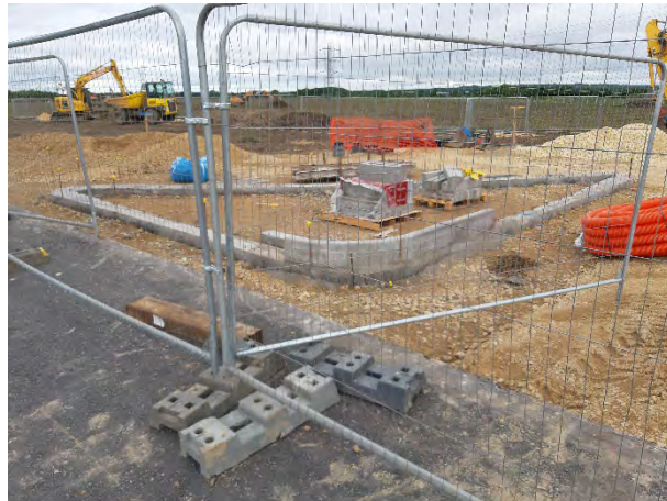
Figure 4. Cast lower section and kerb units to island unit of 278 works on International Drive.
