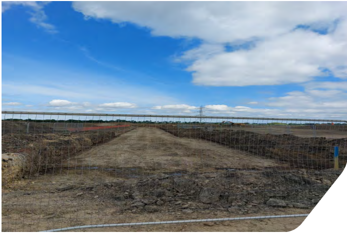
Photo 07: Halted works near vehicle entrance of A1290
