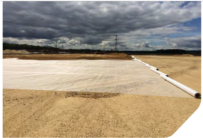
Photo 10: Placement of second geotextile membrane over type 1 forming the piling matt in Zone 2.
