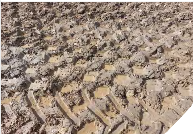
Photo 05: Water retained on surface in padfoot wells in Zone 8/9
