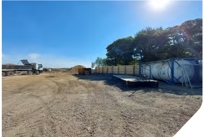
Photo 08: Water tank and compound off vehicle entrance from A1290
