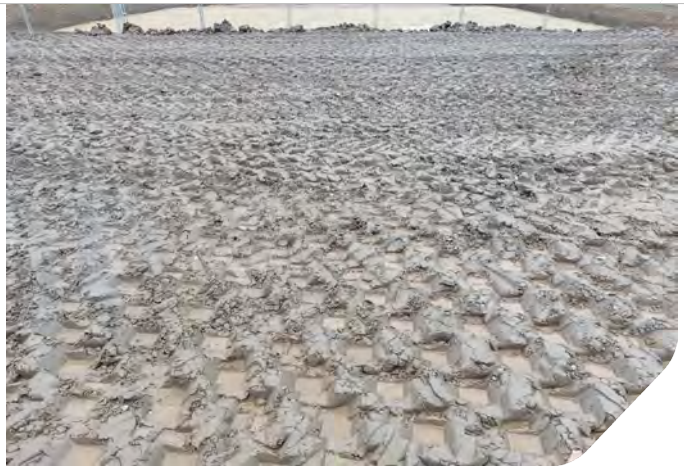
Photo 04: Standing water within padfoot dimples in Zone 6
