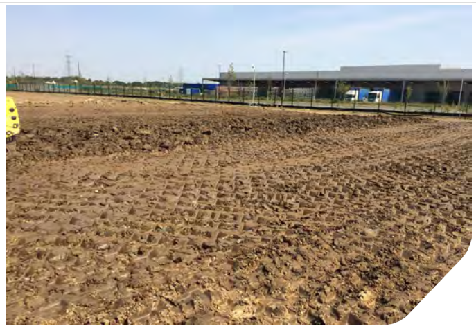
Photo 06: Showing area to be roller by pad foot roller, clearly shows the small areas being rolled to enable moisture to be added due to very hot and dry weather conditions.
