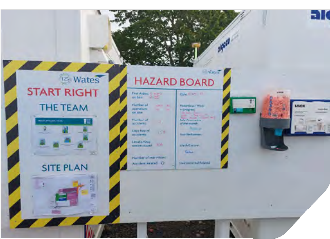
Photo 01: Updated hazard board at Wates compound
