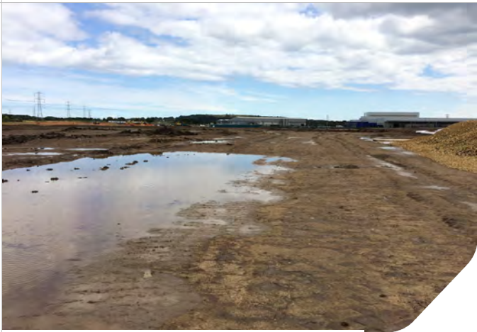
Photo 09: Pooled surface water in zone 6, ponded in the areas of deeper cut.
