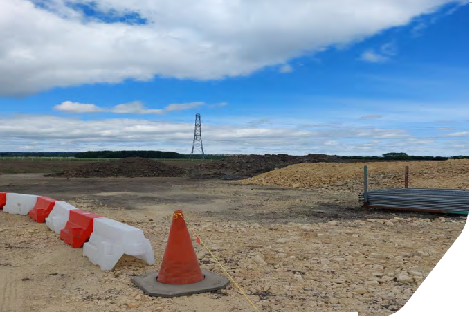
Photo 10: Stockpiles awaiting WAC testing results
