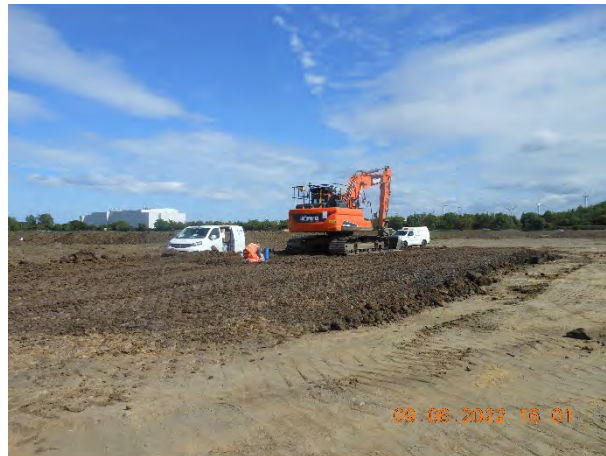
Figure 30. Test pad area following passes three and four during sample taking and testing.
