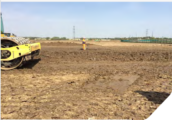
Photo 05: Pad foot roller, area prepared for core cutter test, core cutter test been undertaken.
