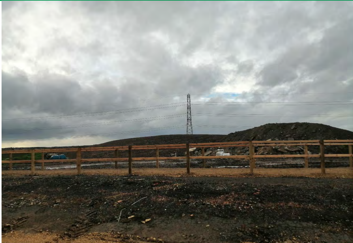
PLATE 3 – CUT SURFACE AND STOCKPILED MATERIALS IN THE SOUTH-WESTERN SITE AREA FOR OFFSITE DISPOSAL
