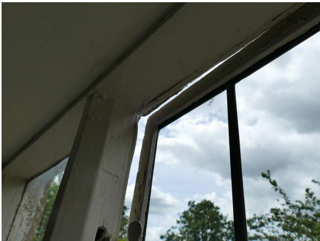
Photograph 10 – Further evidence of metal casement twisted and poorly fitting to timber frame, resulting in clear daylight visible between frame and casement ( First Floor Rear Elevation Window (WF6) )
