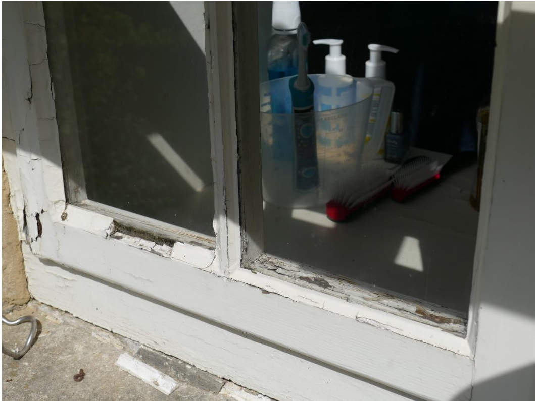
Photograph 19 – Defective missing and cracking window putty Second Floor Front Elevation Dormer Window (WS2)
