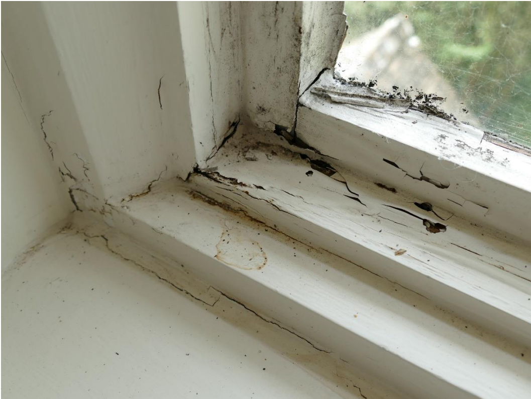
Photograph 21 – Further evidence of severe softening and rot to top side of bottom rail and glazing bars internally (Second Floor Rear Elevation Dormer Window (WS4))
