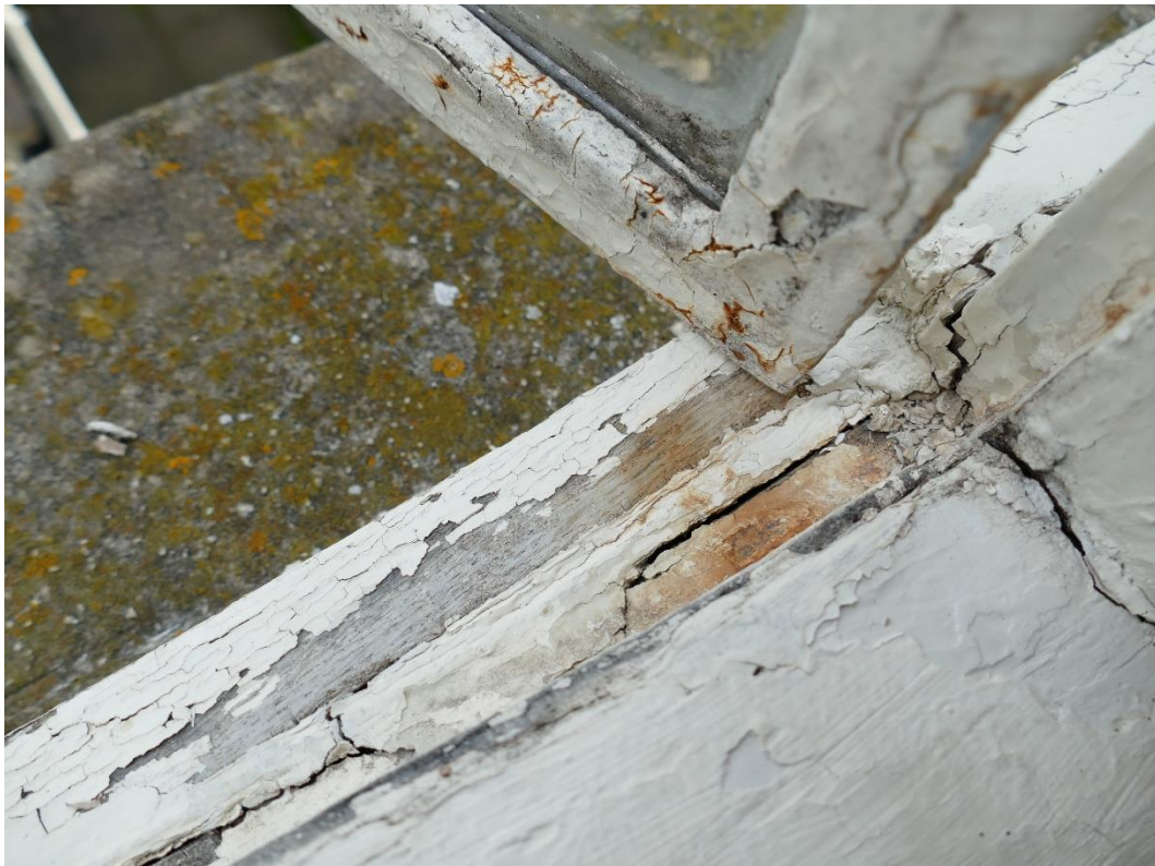
Photograph 12 – Cracking and rot to timber cill, with this particularly evident to opening casement due to rainwater penetration ( First Floor Rear Elevation Window (WF6) )
