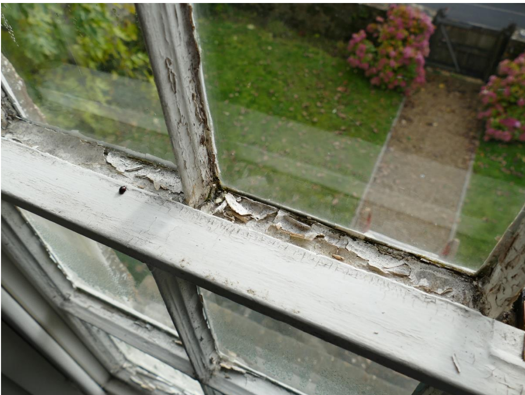
Photograph 8 – Defective peeling/flaking paint to on-set of rot to glazing bars to a sliding sash window as visible internally ( First Floor Front Elevation Window (WF2) )
