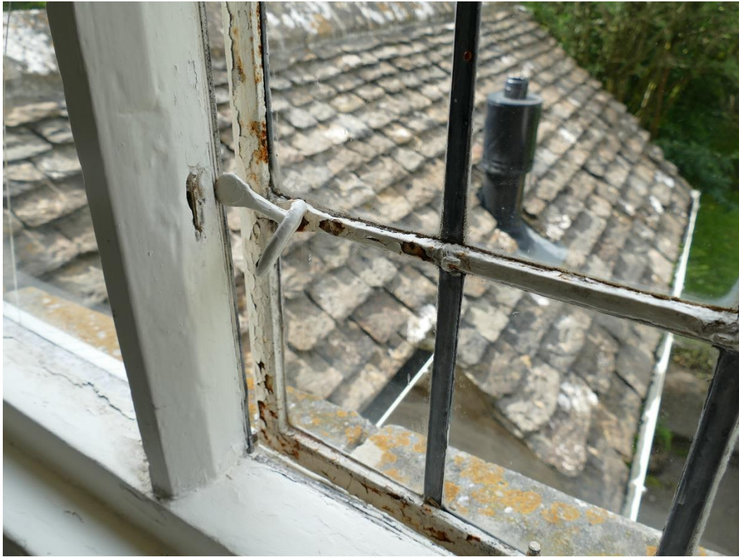
Photograph 11 – Further evidence of poor condition of metal casement, with rust, defective sash fastener and inability to close window ( First Floor Rear Elevation Window (WF6) )
