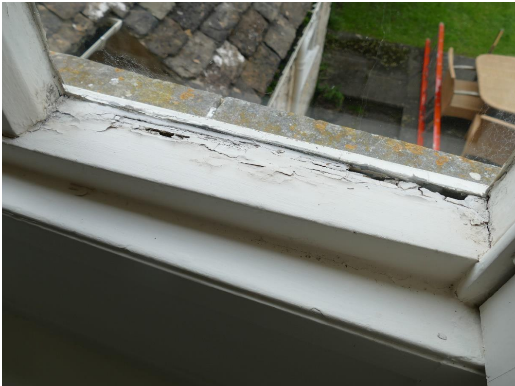
Photograph 14 – Further evidence of cracking and rot to timber cill internally First Floor Rear Elevation Window (WF6)
