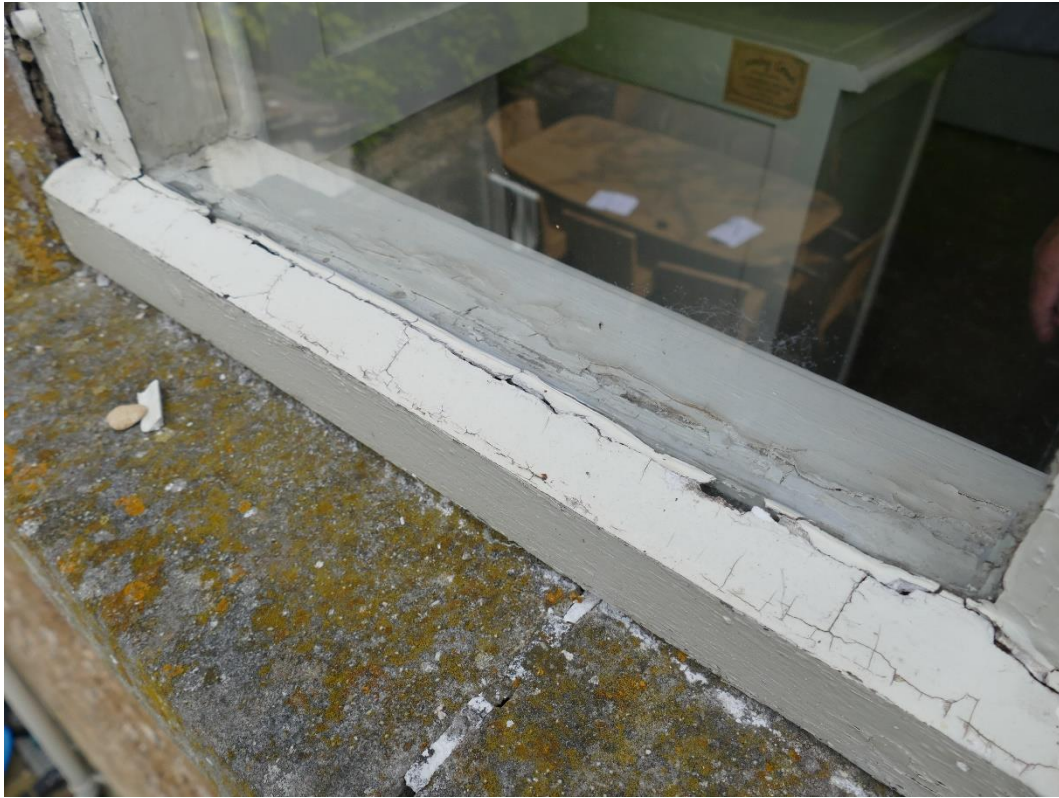
Photograph 13 – Further evidence of cracking and rot to timber cill First Floor Rear Elevation Window (WF6)
