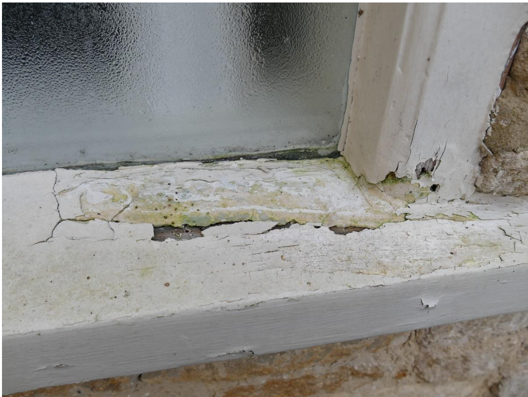
Photograph 16 – Rot and deterioration to cill and jamb to top-hung fanlight Ground Floor Rear Elevation Window (WG8)
