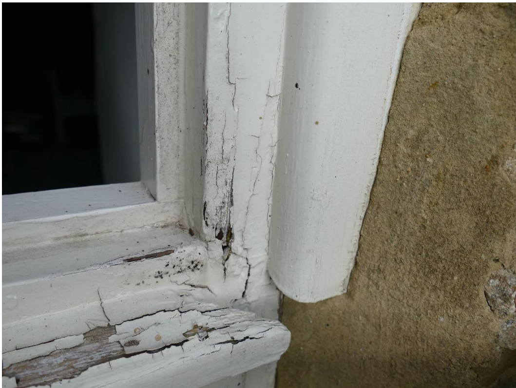
Photograph 18 – Severe rot to right-hand jamb and transom (with equal severe rot to mullion and cill not shown) ( Second Floor Front Elevation Dormer Window (WS3) )
