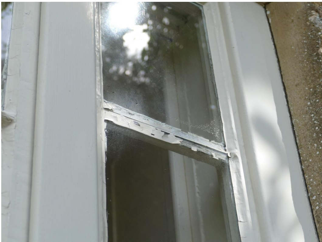
Photograph 6 – Further evidence of completely missing glazing bar to fixed sash casement First Floor Front Elevation Window (WF3)
