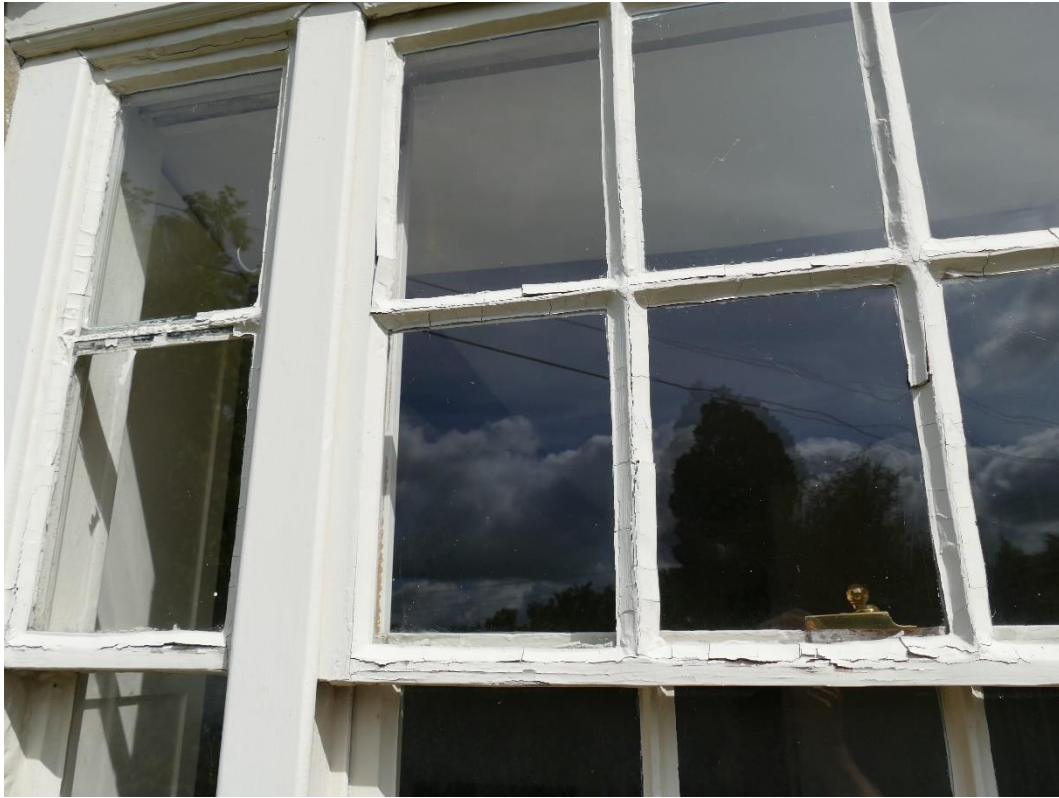
Photograph 5 – Defective rotten and missing glazing bar, with missing and cracking window putty ( First Floor Front Elevation Window (WF1) )
