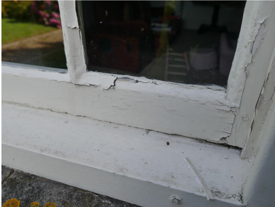
Photograph 1 – Softening and on-set of rot to right-hand side bottom rail to lower sliding sash at abutment with stile ( Ground Floor Front Elevation Window (WG2) )
