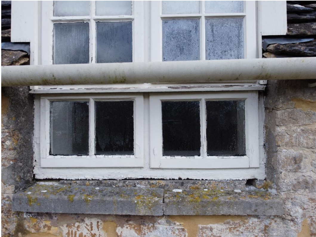
Photograph 17 – General poor condition of dormer window, with defective peeling/flaking paint, rot and cracking/defective window putty ( Second Floor Rear Elevation Dormer Window (WS4) )
