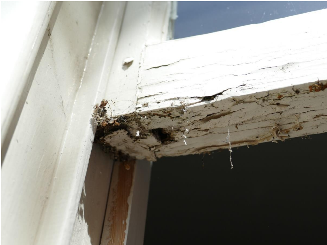
Photograph 4 – Rot to face and soffit of bottom rail to lower sash externally at intersection with stiles on carpentry joint ( First Floor Front Elevation Window (WF3) )
