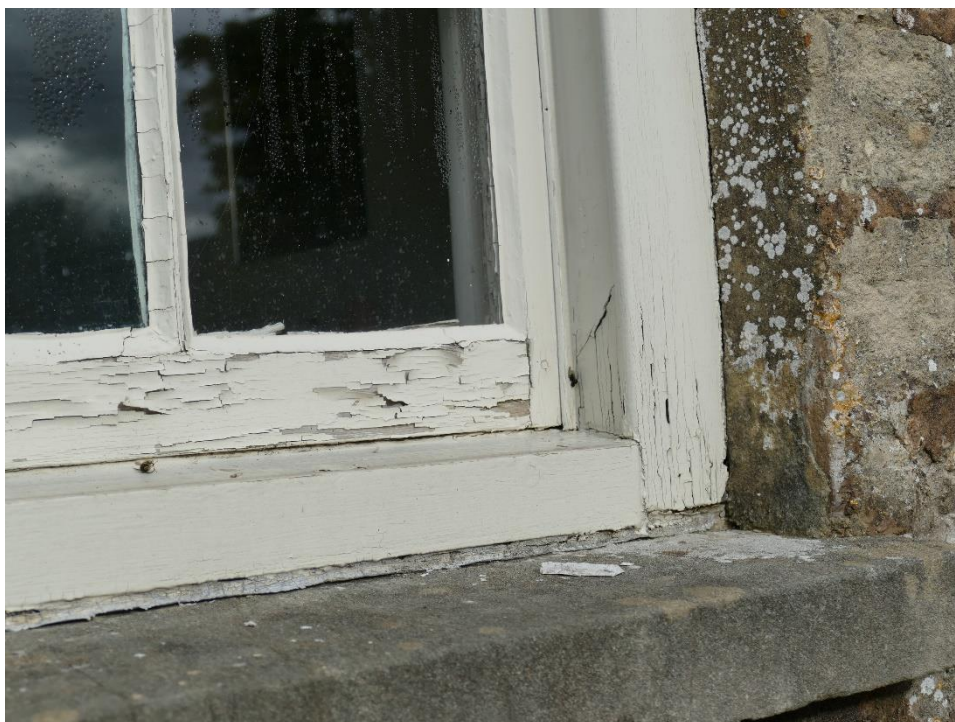
Photograph 2 – Defective peeling/flaking paint, softening and on-set of rot to bottom rail, outer lining, parting beads and pulley stile – despite splice repairs ( First Floor Front Elevation Window (WF2) )
