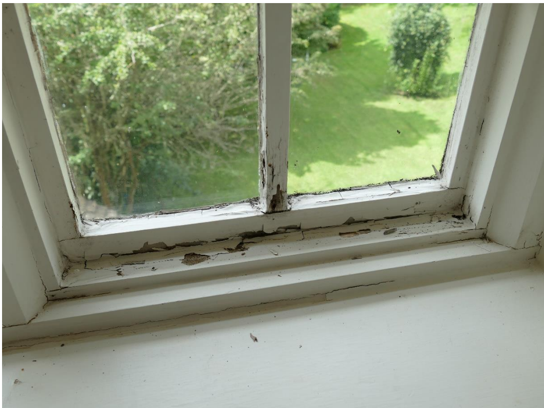
Photograph 20 – Severe softening and rot to top side of bottom rail and glazing bars internally Second Floor Rear Elevation Dormer Window (WS4)
