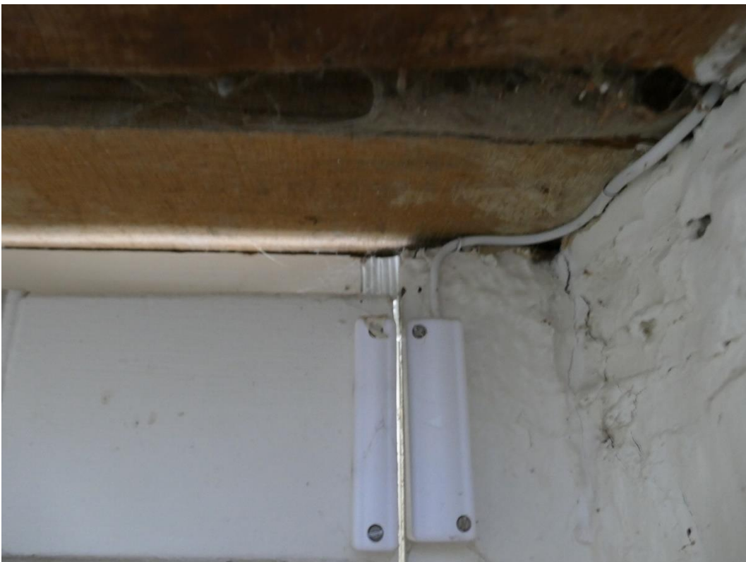
Photograph 22 – Clear daylight visible between the door and frame to the kitchen (DG2), despite the presence of draught stripping, as a result of the twisting of the door
