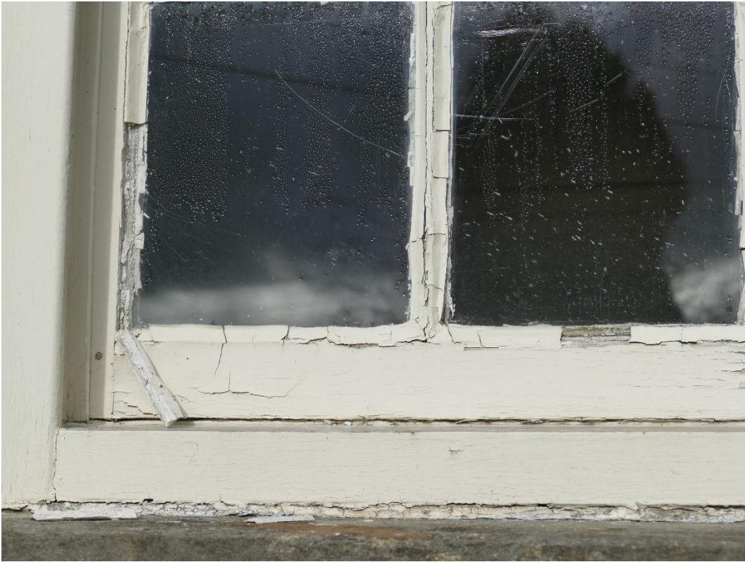
Photograph 7 – Further evidence of defective missing and cracking window putty First Floor Front Elevation Window (WF2)
