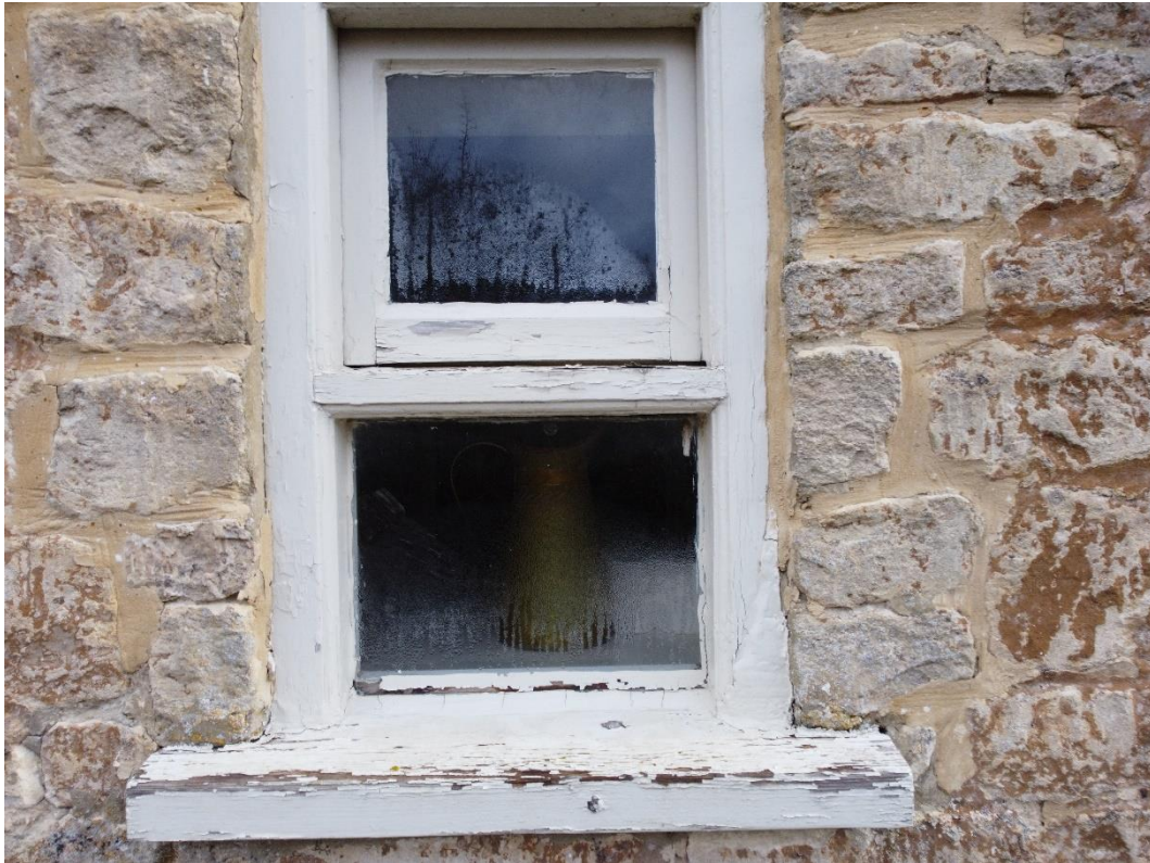
Photograph 15 – Severe poor condition of top-hung fanlight, with severe rot throughout including to: transom, cill, head of frame, bottom rail to fanlight First Floor Rear Elevation Window (WF7)
