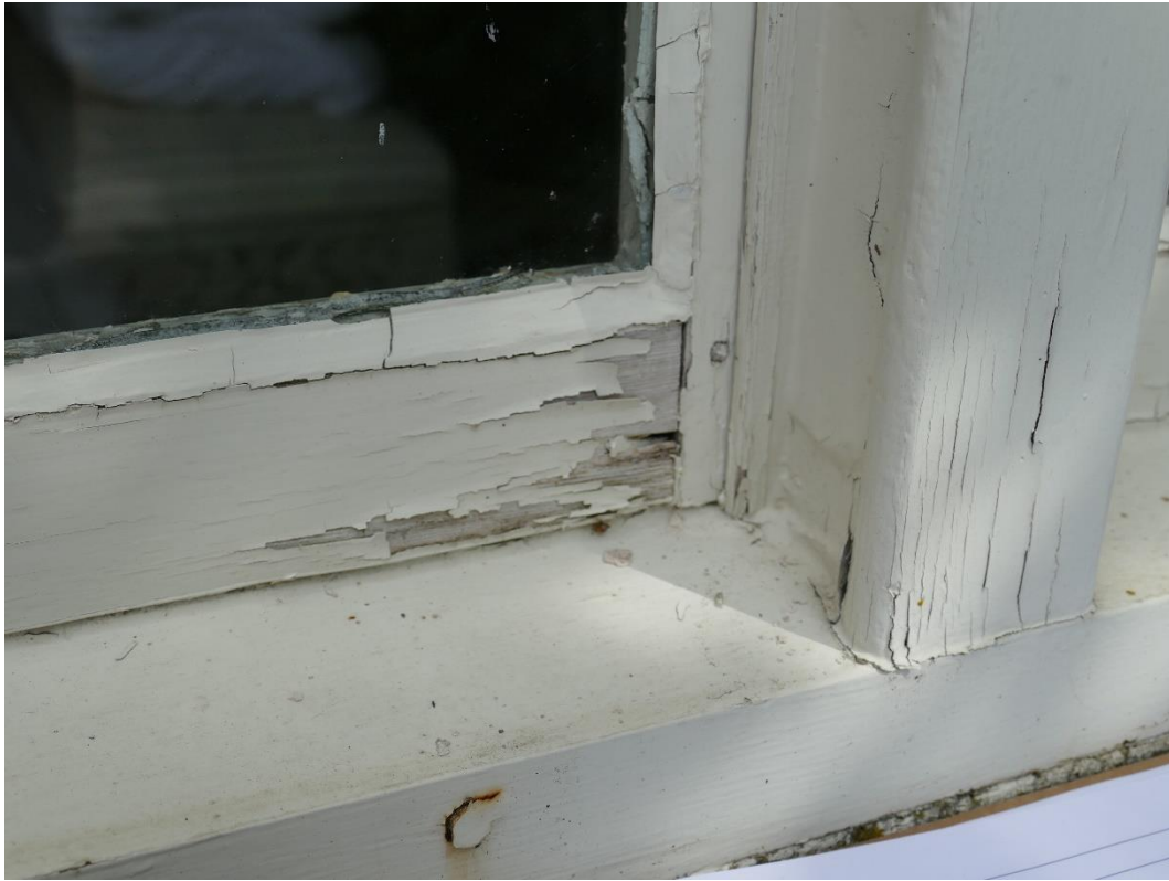
Photograph 3 – Defective peeling/flaking paint, rot to bottom rail, outer lining, parting beads and pulley stile ( First Floor Front Elevation Window (WF3) )
