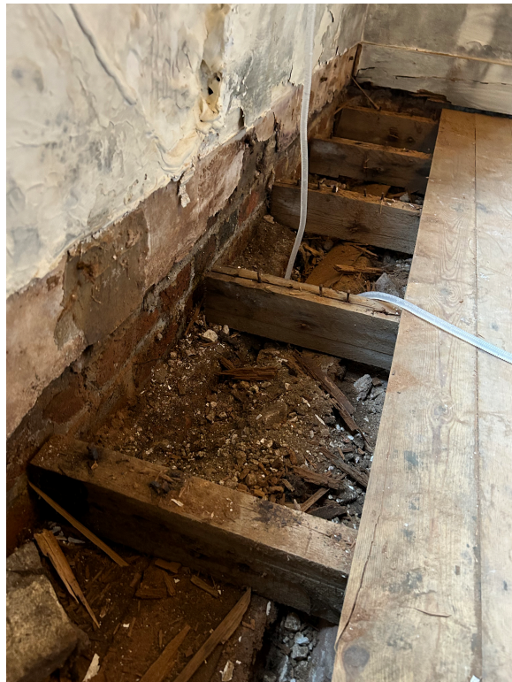
No ventilation to floor and extensive decay to sole plate.
