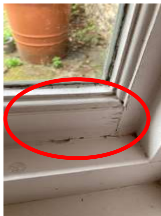
Frame Deterioration & Rot
