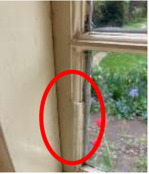
Multiple poorly spliced repairs
