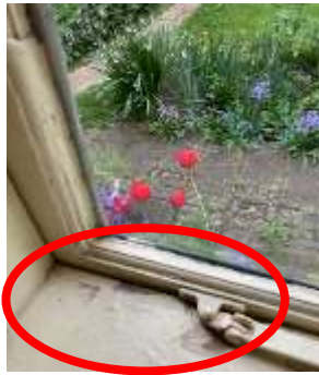
Gapping, frame deterioration
