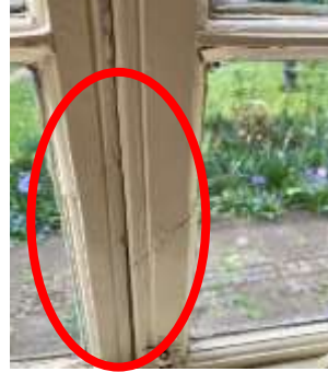
Multiple poorly spliced repairs
