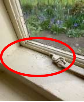
Gapping, water ingress
