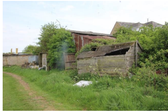
10. The collapsing chicken coop
