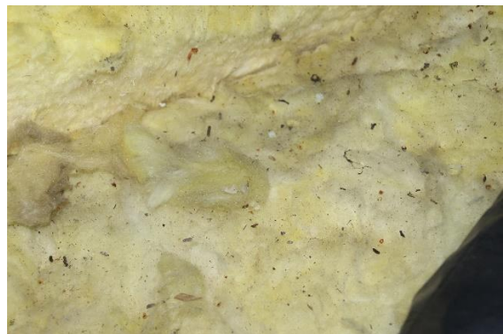
12. Bat droppings on fibreglass
