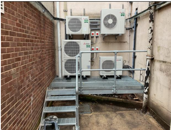
Figure 4 Installed condenser units
