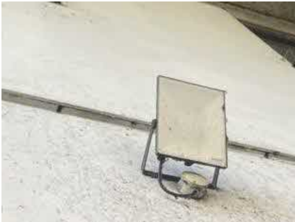
Photo 7: Security Light and Ventilation Gaps on the Eastern Side of B1a
