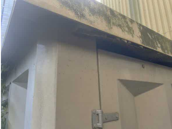
Photo 36: Gap Under the Eaves on B3
