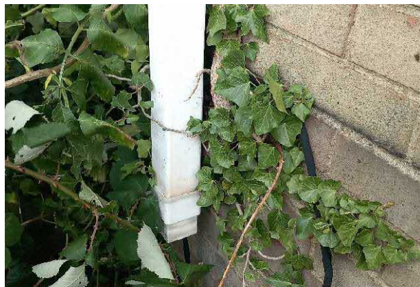
Photograph 7: View of disconnected front downpipe
