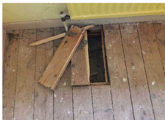
Photograph 15: View of timber flooring with broken floorboards
