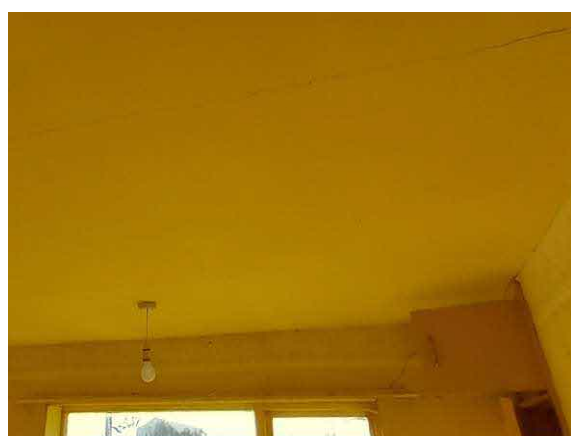
Photograph 17: View of cracking in the plasterboard (1)
