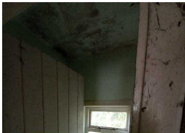
Photograph 9: View of mould growth in a small room of the building
