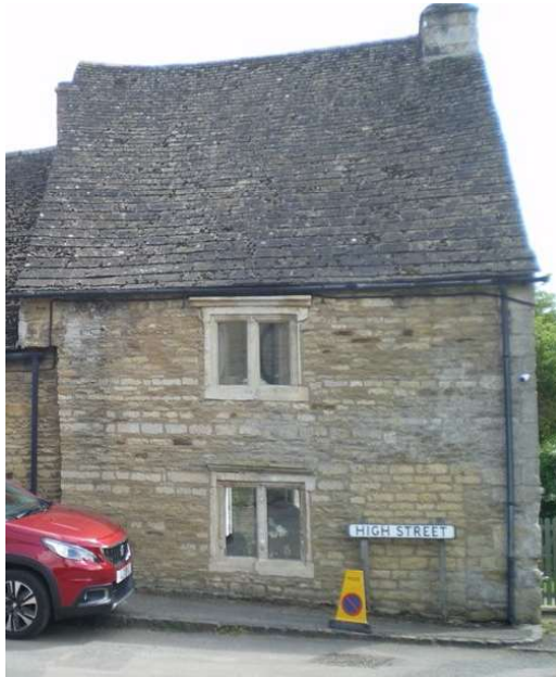
Glazing to be replaced
