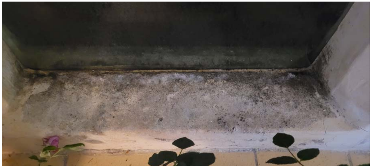
Above: photographs showing the significant amounts of condensation forming on the inside of the windows
