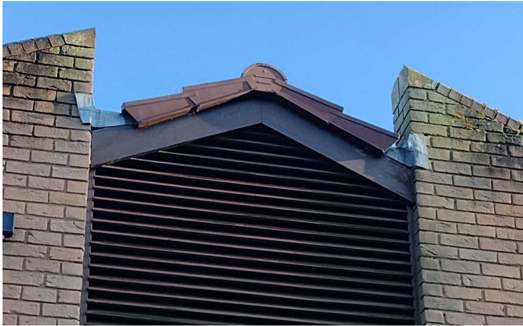
Plate 9: Gaps beneath the lead flashing
