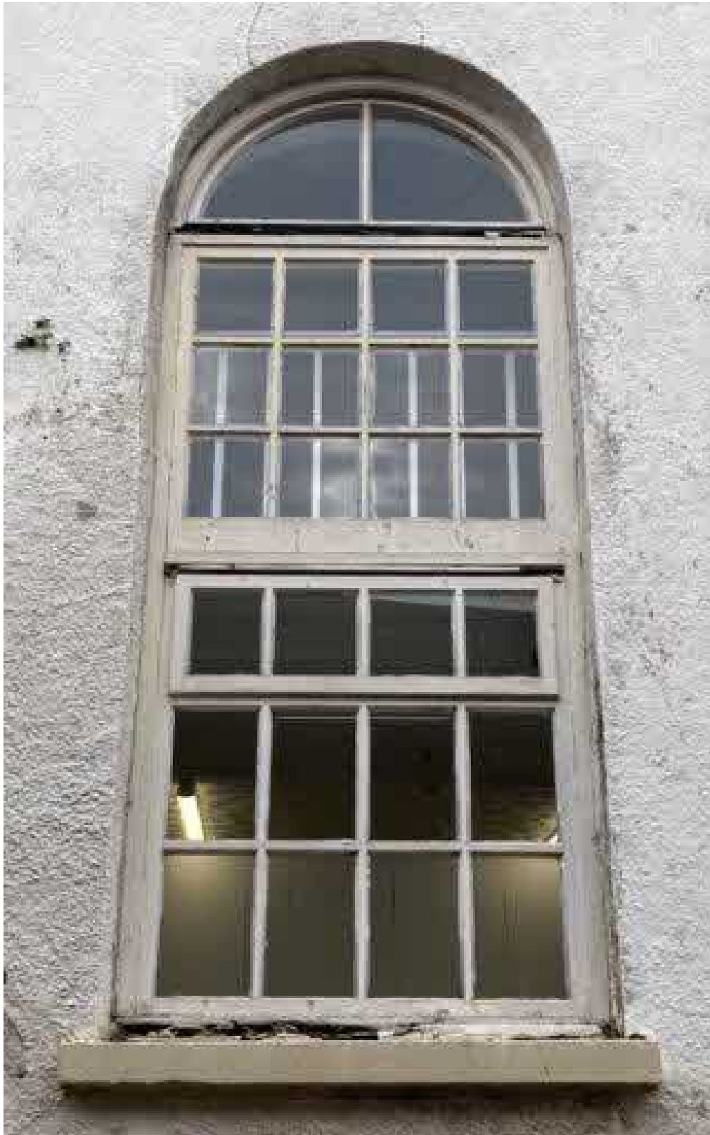
Fig 7 - Windows W.4. and W.9. (South Elevation). Windows W.5. / W.10. and W.6. / W.11. are the same.
