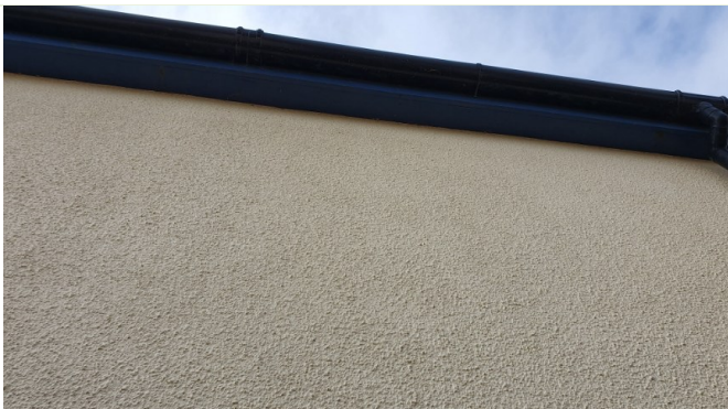
Very tight barge boards throughout
