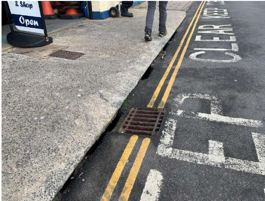
Photo 9. Surface water drains leading to a gully below the concrete entrance ramp
