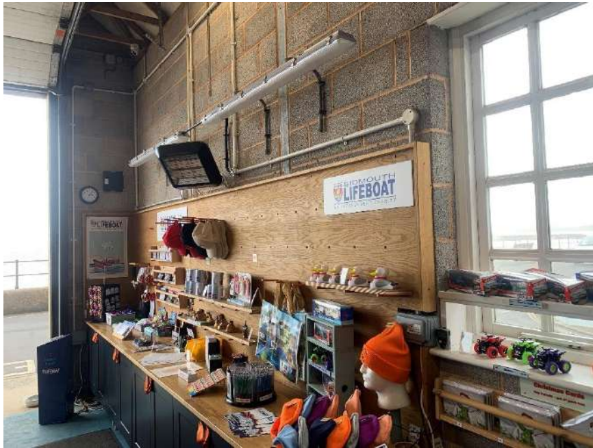
Photo 11. Current internal configuration (note raised, falling electrical fittings and unplastered block work)
