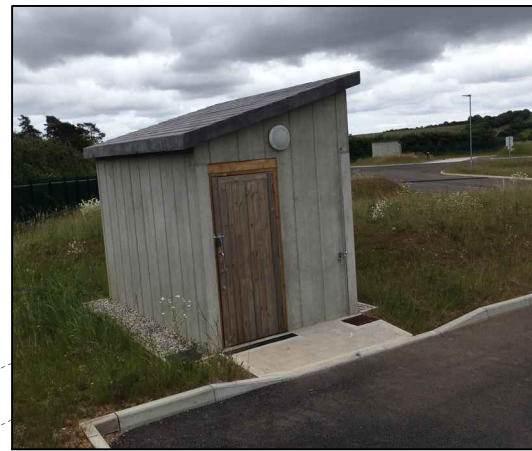
TYPICAL ABLUTION BLOCK: MOULDED CONCRETE TO RESEMBLE SLATE ROOF OVER TIMBER CLADDED WALLS
