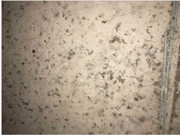
Bat droppings of mixed age – loft room
