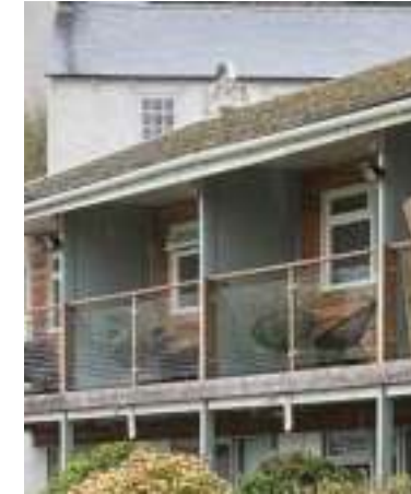
Building mounted flood lighting
