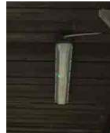
Canopy mounted exterior strip lighting
