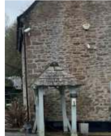
Wall mounted (shielded) spot lighting
