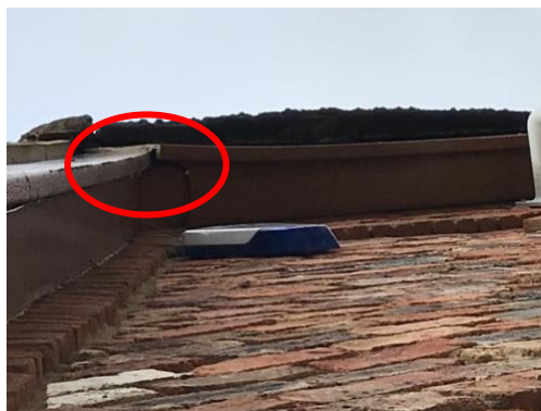
Photograph 12: Gap in the soffit at the apex of the eastern aspect
