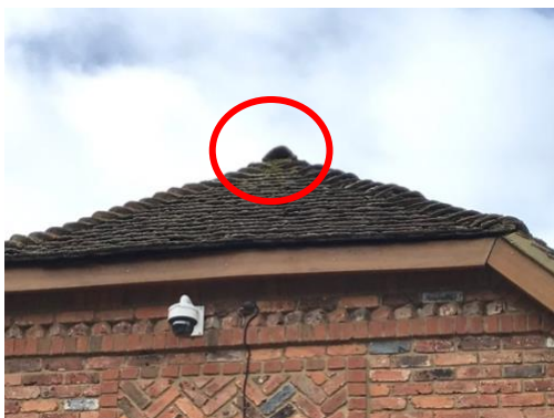
Photograph 11: Missing mortar on eastern aspect of B1
