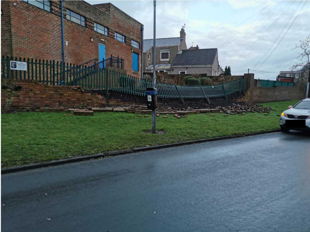
Current state of retaining was after collapse
