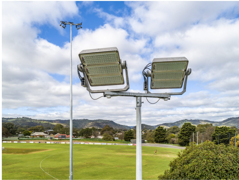
FLOODLIGHT MAST WITH LED LUMINAIRES
