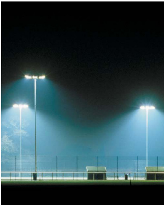
Well directed lighting onto the pitch avoids light pollution into surrounding areas and into the night sky.
