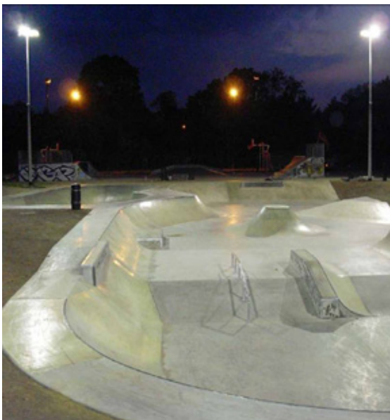
Skate park floodlighting installation using tall columns
