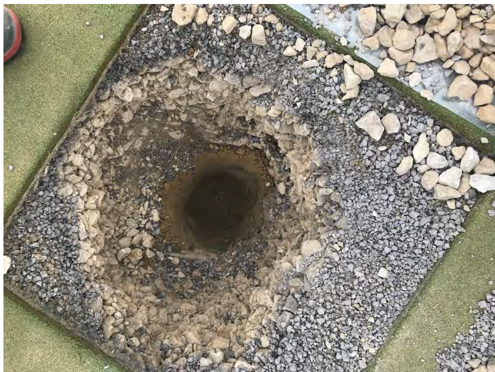
Photograph 3.3.4: cut out through the pitch with hand pit excavation through subbase and subgrade
