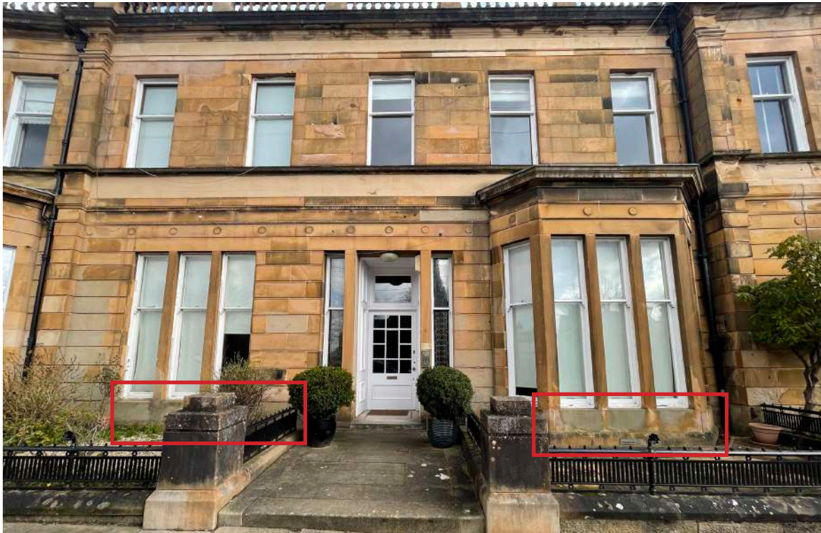
Poorly repaired stone to the front elevation
