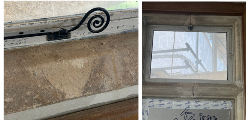
Images above: LHS shows missing mullion. RHS shows structural failures where mullions were removed.
