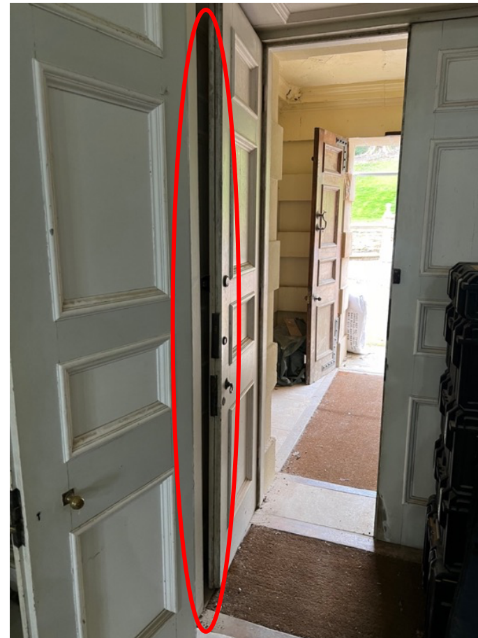
Image of the three doors in succession. Note the gap on the second set of doors, between frame and door. This implies this second set of doors is unlikely to be part of Lutyens' design, clearly diminishing their significance.
