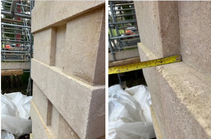
Photos above of porch as standing today. Note the completely flat exposed face, nominally 3" deep, recessed 2" behind the outer face.
