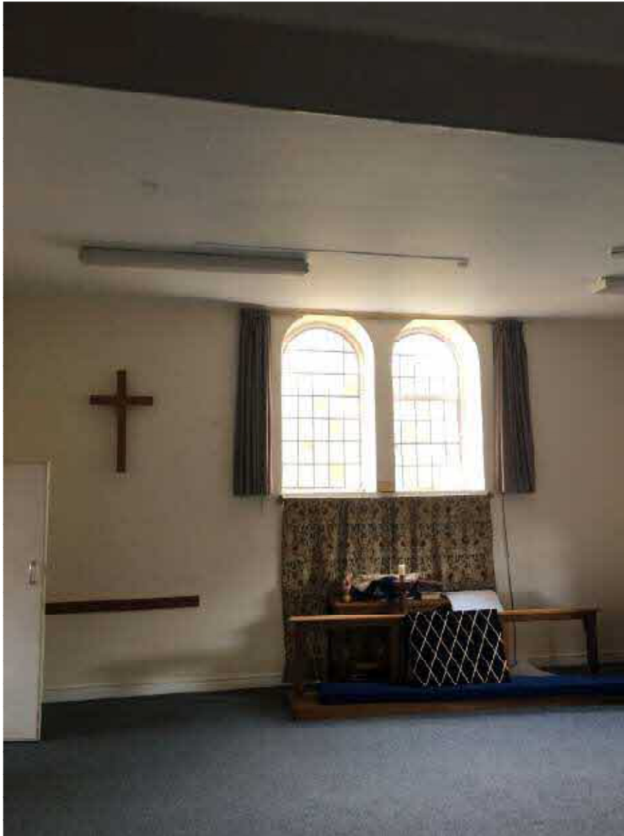
Fig 21: South elevation windows as seen from inside the church, showing false ceiling.
