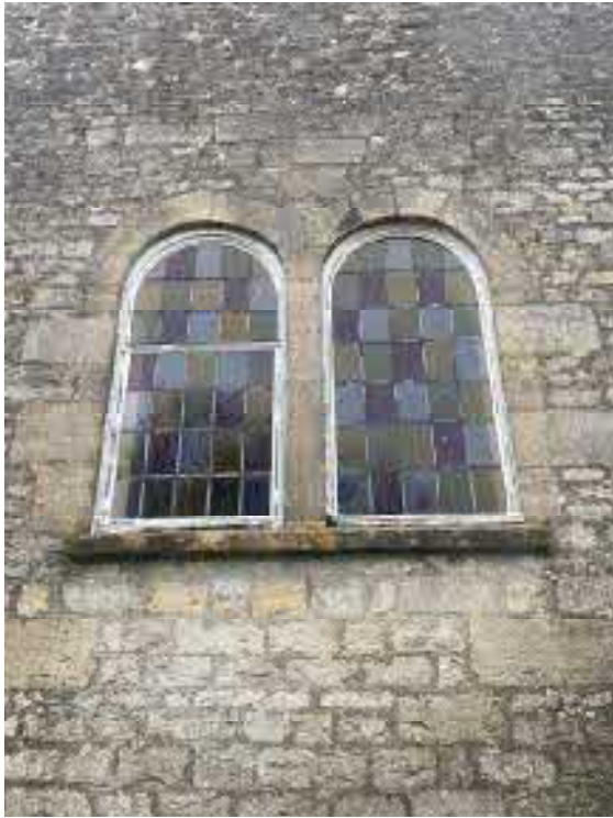
Fig 15: Church windows in south elevation (proposed to be raised to a higher level).
