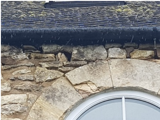
Photo 7: Gaps in stonework to top of wall - west facing elevation
