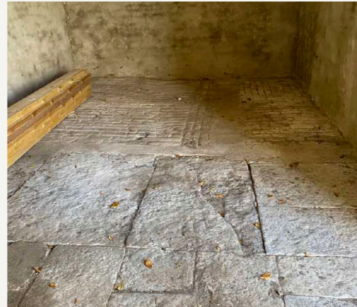
INTERNAL FLAGSTONES SUGGEST TWO SEPARATE BAYS TO AN ORIGINAL BARN. SLABS TO BE RETAINED.
