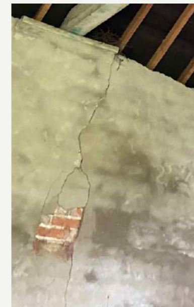
BOWED AND CRACKED WALL BELOW THE ROOF TRUSS
