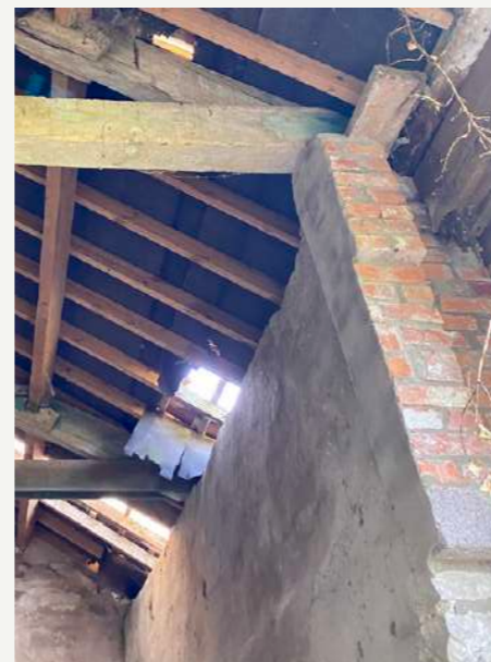
THE BARN ROOF IS BALANCING ON A SMALL BRICK CORBEL
