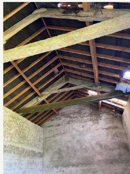
EXISTING ROOF INCLUDES TWO HEAVY ALTERED UNMATCHED TRUSSES AND MODERN RAFTERS
