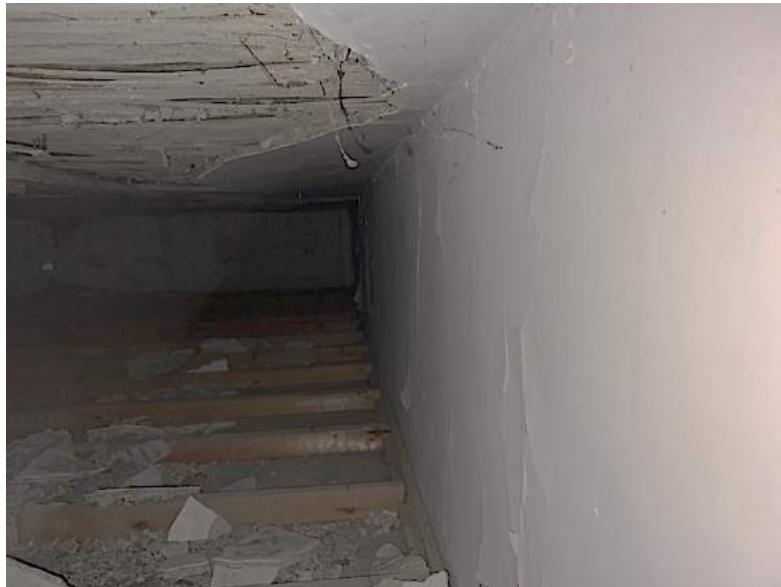
Figure 97 Void between modern false ceiling, & 19 th -century lath-&-plaster ceiling.
