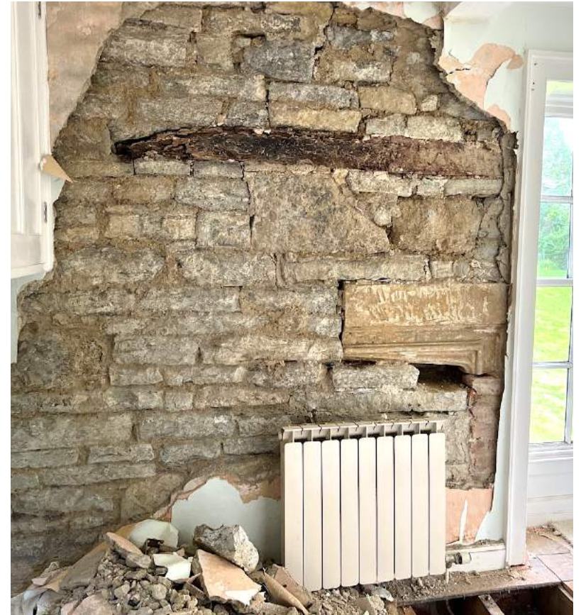
Figure 83 North-east room, east wall, showing the right half of the fireplace head, & a relieving beam above.
