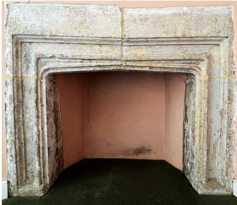
Figure 69 Late-16 th /early-17 th century fireplace in the north-west ordinal projection at second floor.
