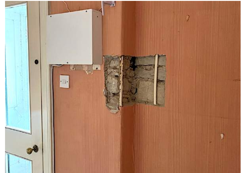
Figure 58 Hall, detail of step in external wall thickness to north of west door.
