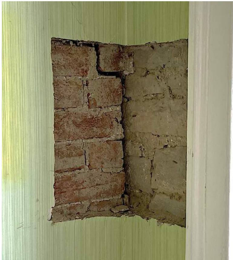
Figure 77 Junction of brick wall dividing the two southern rooms (left) & the inner face of the south elevation.
