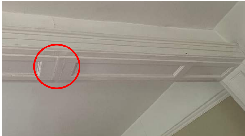
Figure 64 Soffit of drawing room archway, showing scar of alteration.
