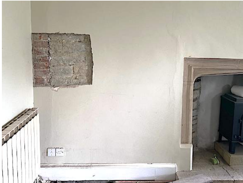
Figure 59 Drawing room, detail of step in wall thickness of eastern elevation (infilled with 19 th -century brickwork).
