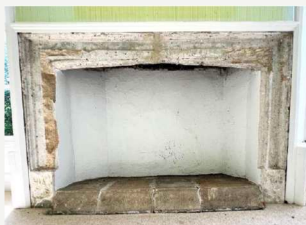
LATE-16TH/EARLY-17TH CENTURY FIREPLACE IN THE SOUTH-WEST ROOM AT FIRST FLOOR TO BE RETAINED - LATER RAISED HEARTH TO BE REMOVED
