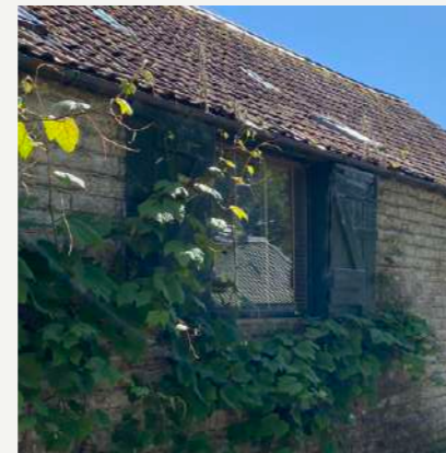
C EXISTING MODERN TIMBER FRAMED WINDOWS TO BE REPLACED WITH NEW CASEMENT WINDOWS
