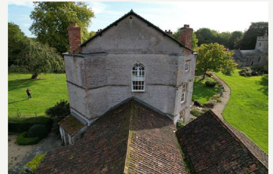
AERIAL VIEW OF THE ROOFS CLOSEST TO THE HOUSE ENCROACHING ON THE MAIN HOUSE
