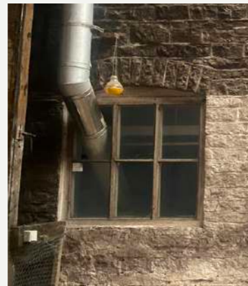
B DAMAGED EXISTING TIMBER CASEMENTS REPLACED WITH NEW TIMBER SILLS WITHIN EXISTING STONE ARCHED LINTELS
