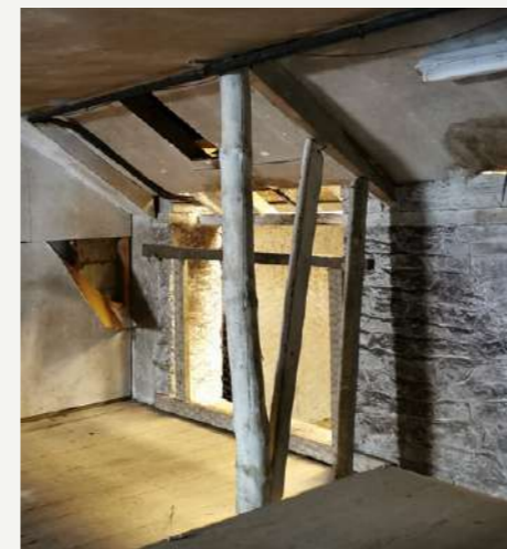
APPLE BARN FIRST FLOOR - TEMPORARY SUPPORTS FOR THE FAILED ROOF
