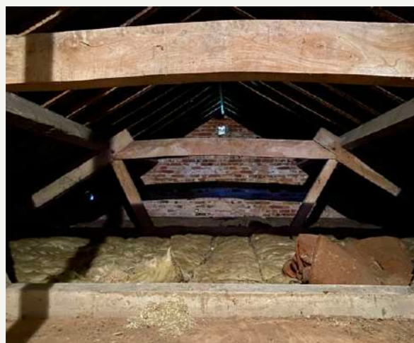
MISSING ROOF RIDGE BEAM RESULTING IN LATERAL THRUST ON THE STONE WALLS
