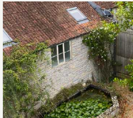
A EXISTING TIMBER CASEMENT WINDOWS IN POOR CONDITION TO BE REPLACED WITH NEW DOUBLE GLAZED TIMBER CASEMENTS IN EXISTING OPENINGS WITH REPLACEMENT TIMBER LINTELS
