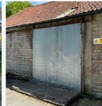
E EXISTING LARGE OPENING TO BE RETAINED, INCLUDING ORIGINAL LINTEL. SILL DROPPED TO MEET INTERNAL FFL, NEW GLAZED INFILL, DOOR AND EXTERNAL SHUTTER.
