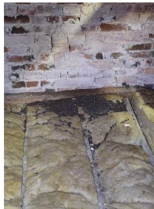
Figure 21, "Bat droppings in main house attic"
