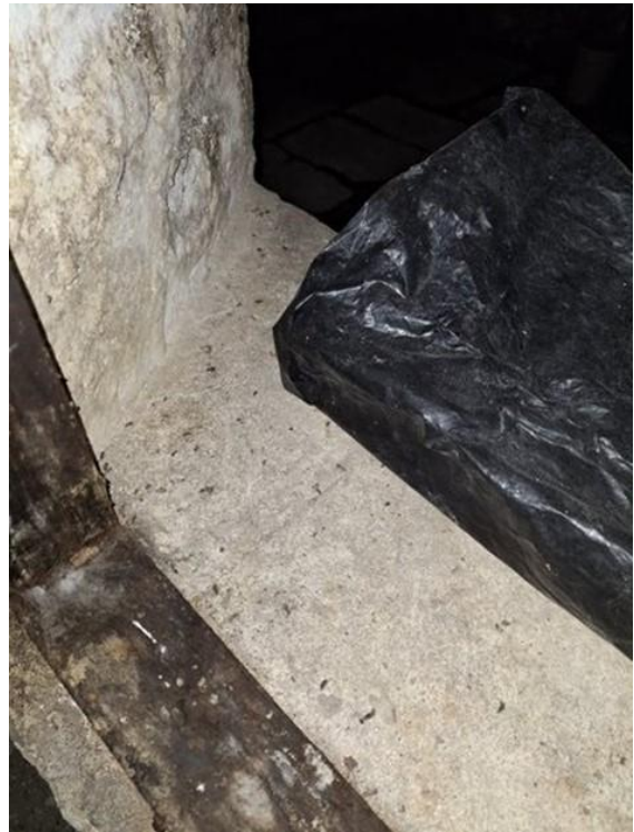
Figure 23, "Droppings in cellar"
