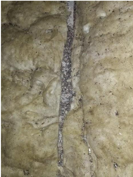
Figure 22, "Droppings under ridge in attic"
