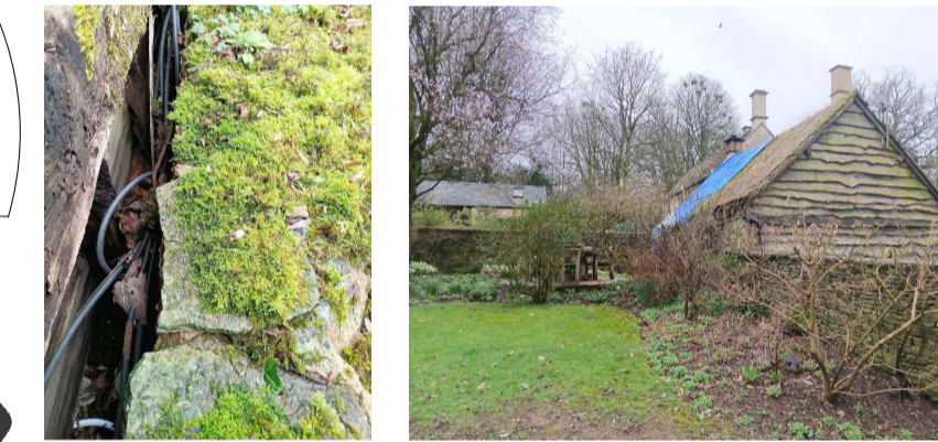
Retaining walls constructed in the 1980's to be modified to suit proposals.
