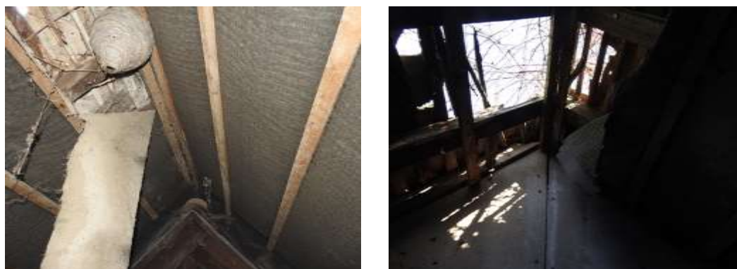
Figs. 15 & 16 Cobwebbed ridge and hole in the roof
