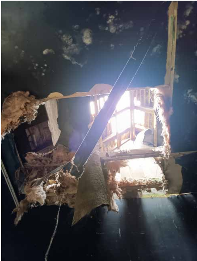
3.16 Detail of perished ceiling and roof in garage (DIA)
