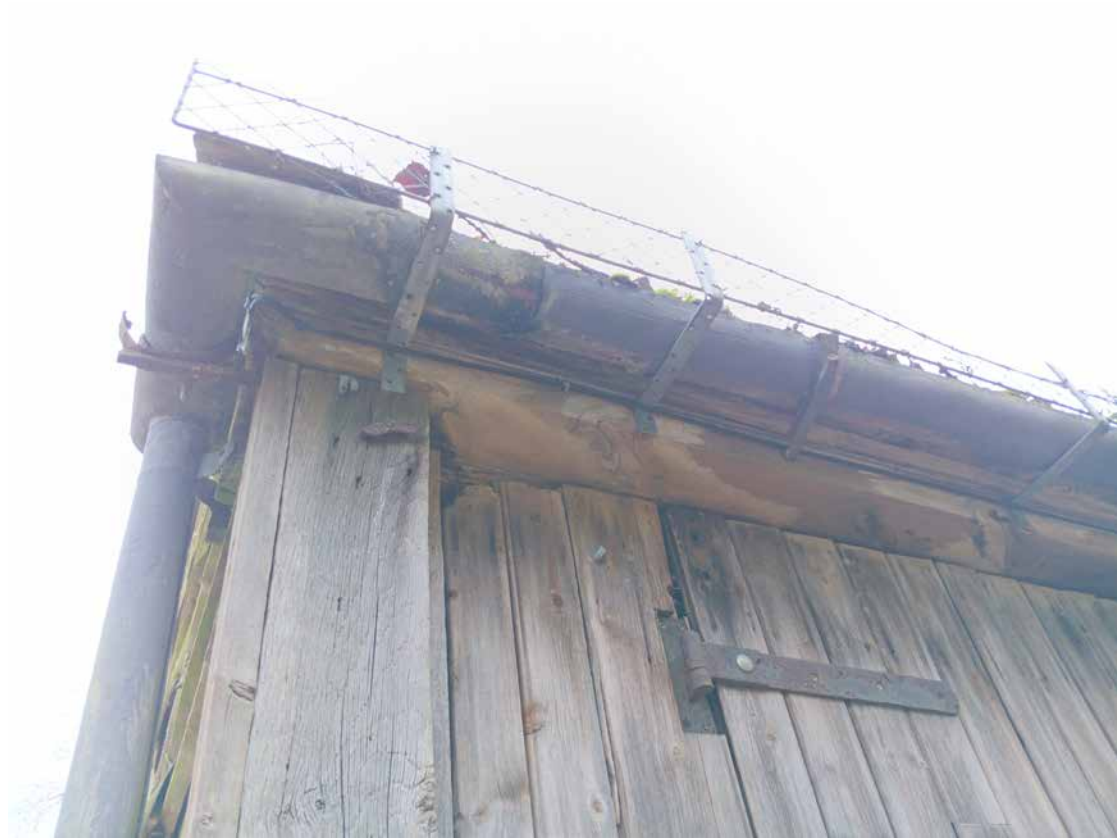
3.15 Detail of failing rainwater goods on garage roof (DIA)
