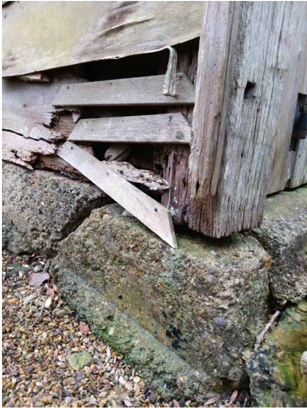
3.14 Detail of deteriorated weatherboarding and post (DIA)
