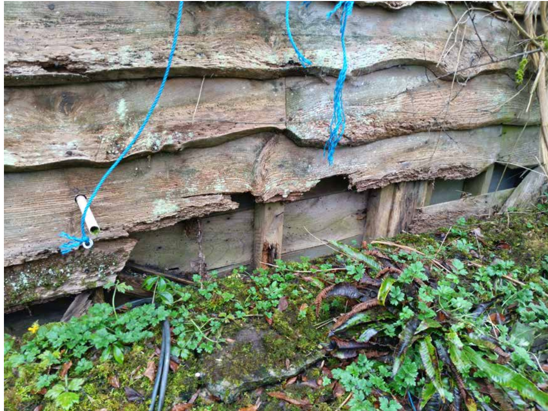
3.17 Detail of rotten weatherboarding (DIA)
