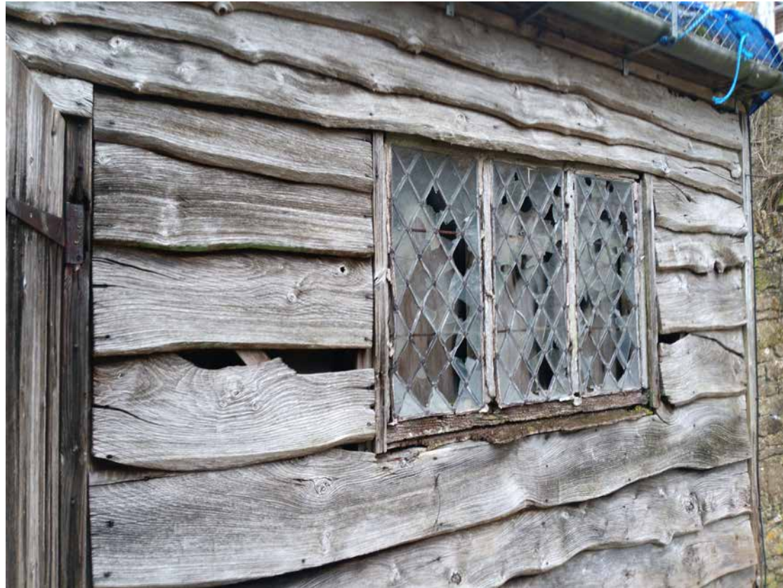
3.8 Detail of modern broken panes and deteriorated weatherboarding (DIA)
