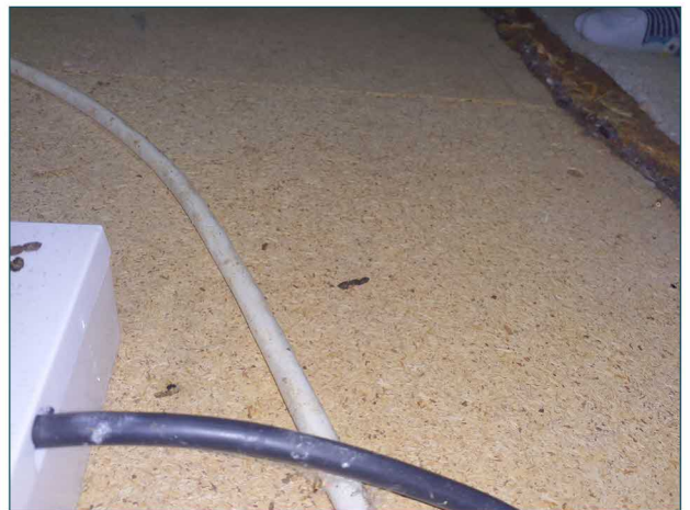
Photograph 12. Single bat dropping, located west gable end of attic space.
