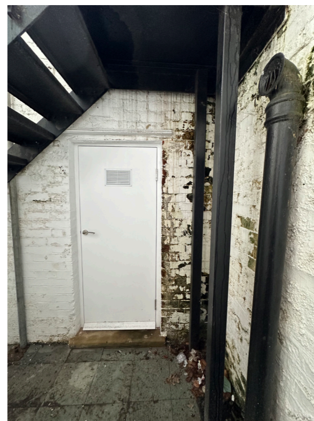
Vault Door, D.LG.15
