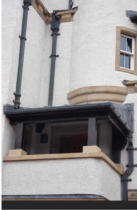
Figure 17 – traditional stone, render and leadwork – extension SE elevation first and second floors – the modulation of planes
