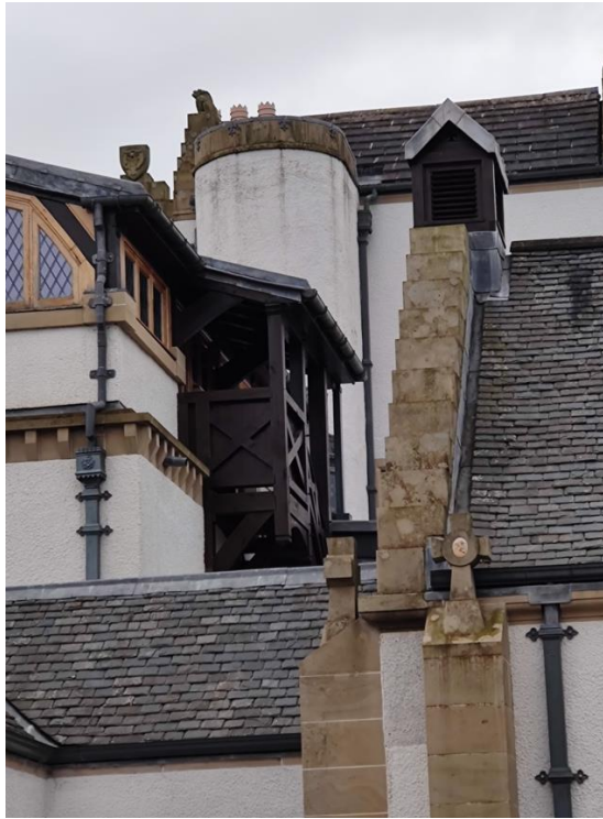
Figure 30 – looking to north east elevation from pool/ chapel courtyard -stepping down in scale, layering of planes and materials
