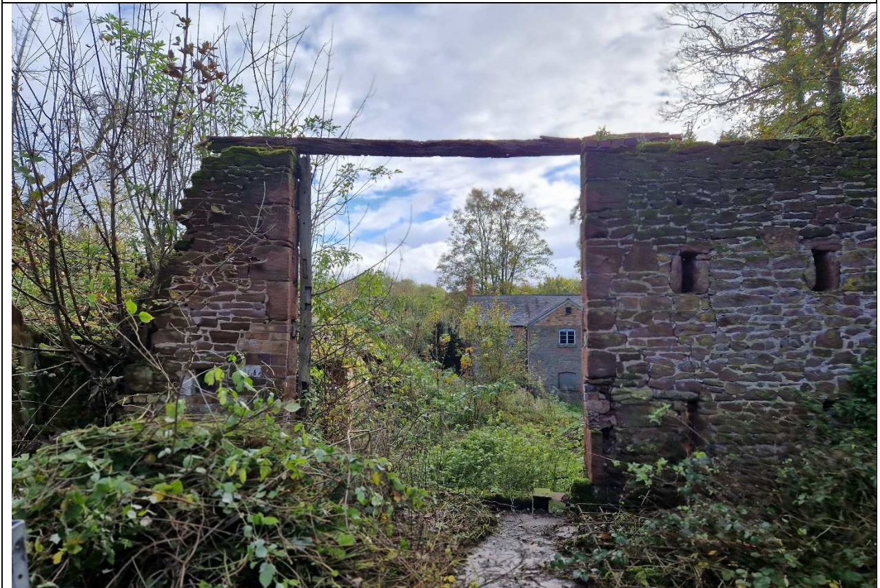
Rear Old Barn Wall With Large Opening
