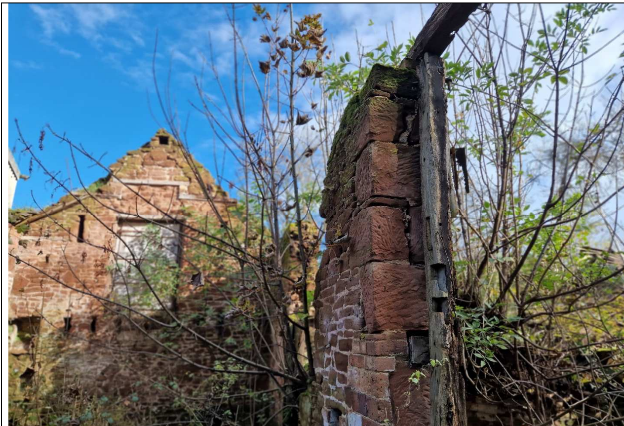
Partial Collapse and Lean to Rear Wall of Old Barn
