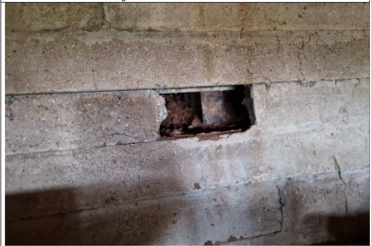
Void in Retaining Wall to Rear Wall
