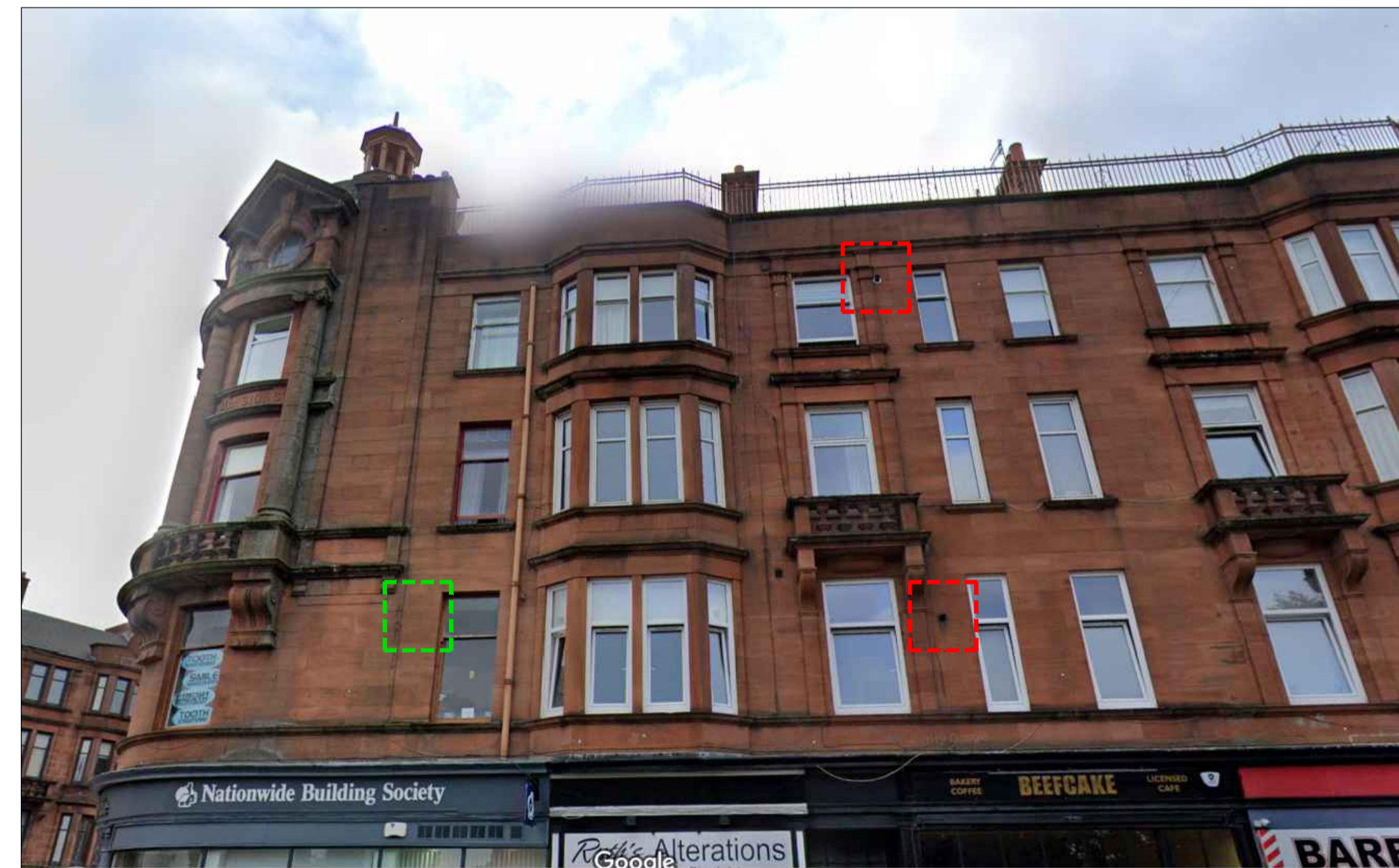
Ventilation Extract Ducts
