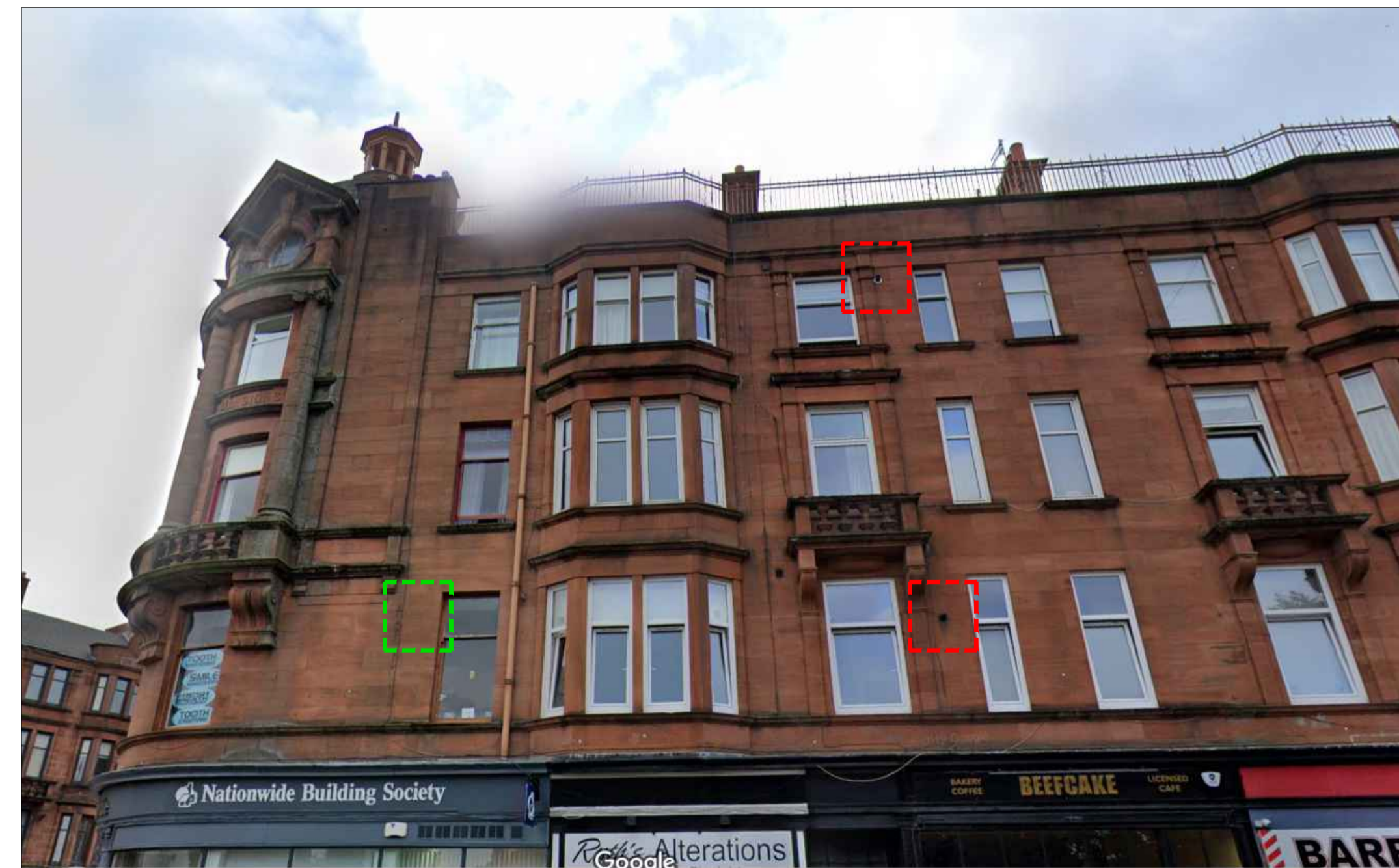
Ventilation Extract Ducts
