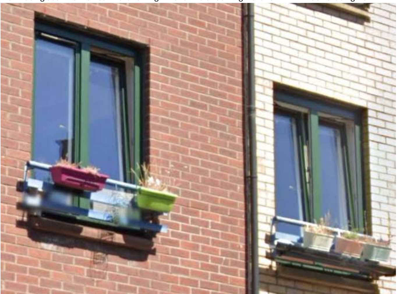
Typical Existing Timber Tilt and Turn Windows (per items 1&2 on the attached schedule) to the Front Elevation of 25 Turnbull Street Glasgow G1 5PR to be Replicated in Size, Configuration, Method of Opening, Material, Frame Dimension and Colour to maintain and Enhance the charter of the property all as required by current Planning Policy.
