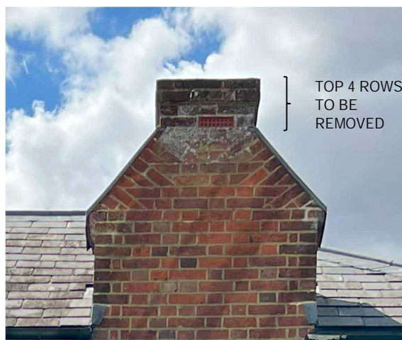
Fig 2: Detail of top of chimney showing which courses are to be removed.
