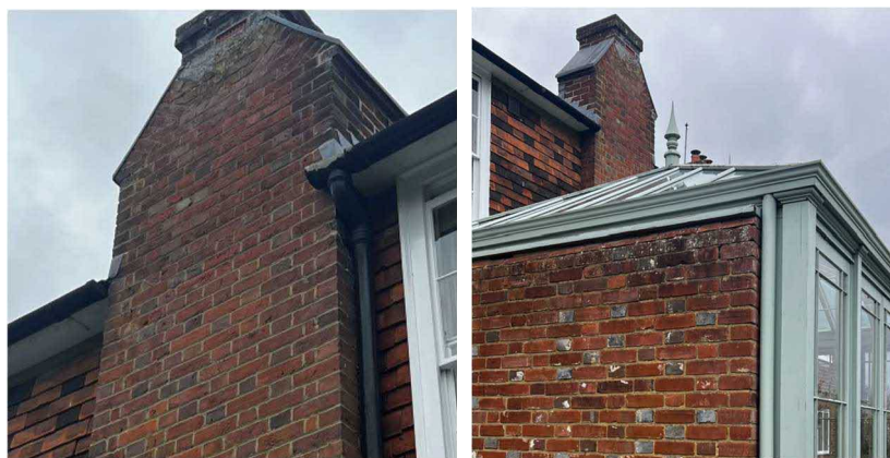
Fig 4: Left –Chimney to be extended, Right –Conservatory to be demolished with chimney in the background
