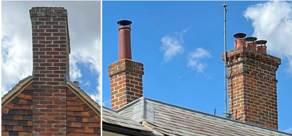
Fig 3: Rear Elevation of Laddingford House showing the existing Chimney's with running bond brickwork
