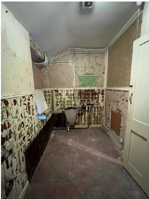
Existing wc – this is proposed to become the children's toilets for the creche
