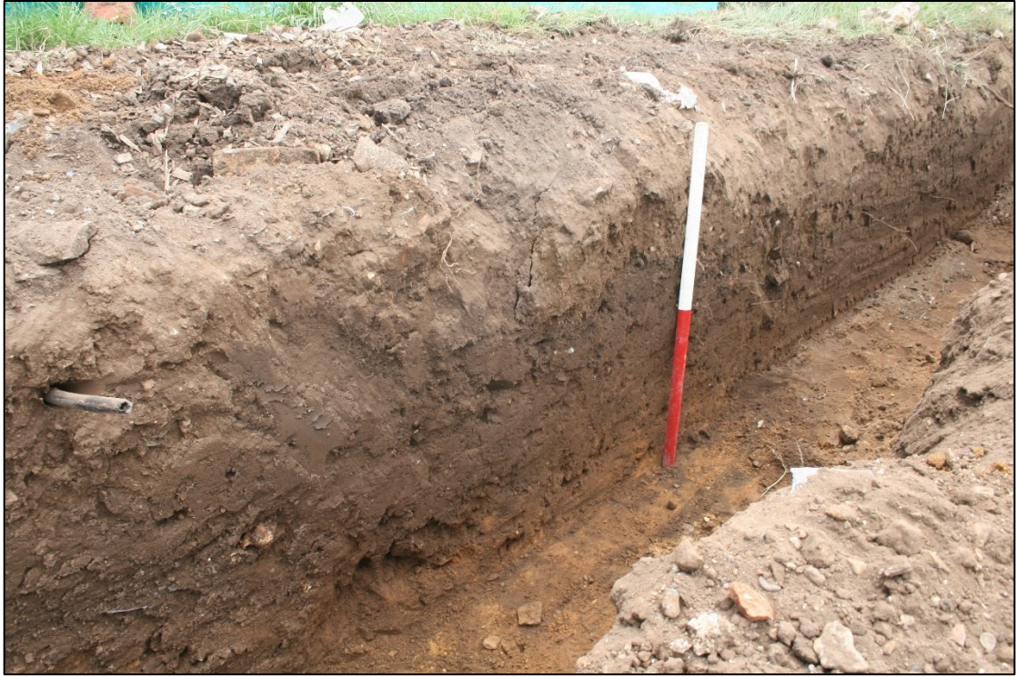
Plate 7: Oblique shot of west facing representative section in north-east of house foundation trench. Fig. 5, sec. 4. Scale 1 x 1m.
