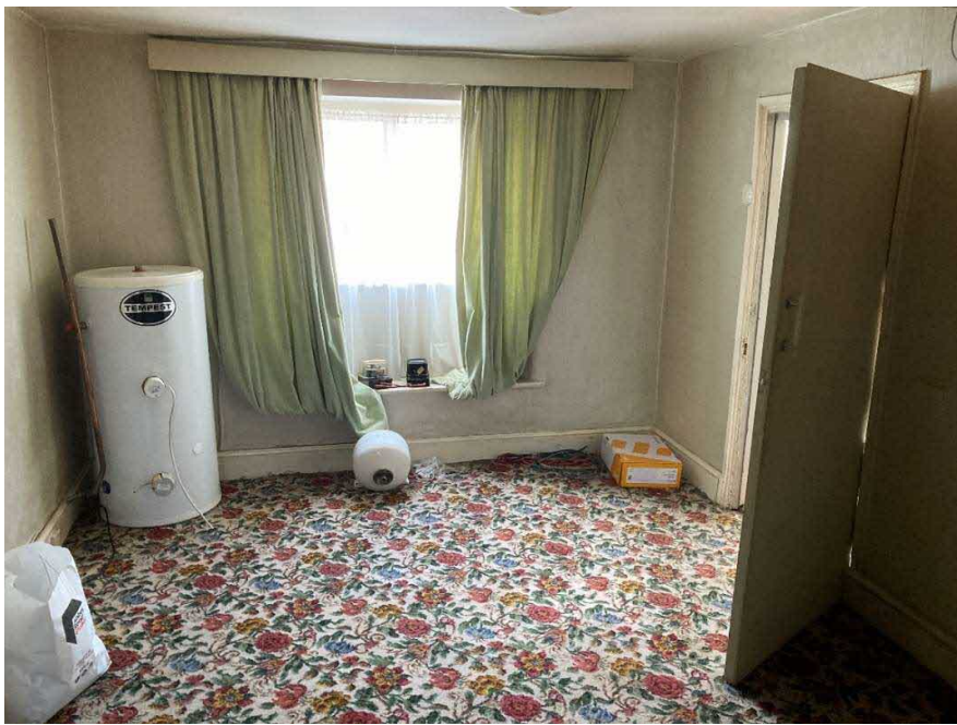
Figure 18. Front room of 18 th -century cottage, looking to front window. There is no sign of the chimney seen in the room above (Figure 24).
