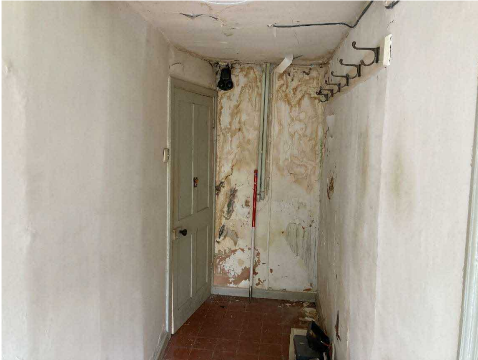
Figure 19. Looking in from the front door of the 18 th -century cottage. The stud wall on the right is original reed and plaster. The door leads into the heated main room.
