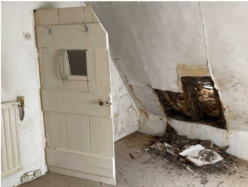
Figure 25. The 19 th -century door into the same room. No 18 th -century joinery survives.
