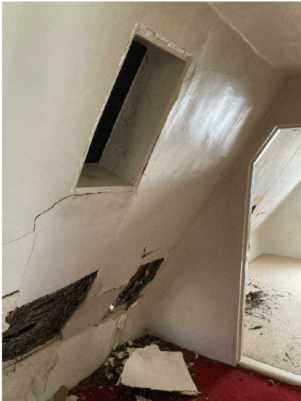
Figure 27. The small window lighting the same passage. Below some plaster has fallen of its reed backing.
