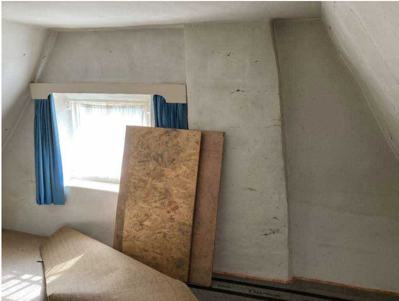
Figure 24. The east wall of the 18 th -century cottage, with a chimney flue, not visible downstairs or externally.
